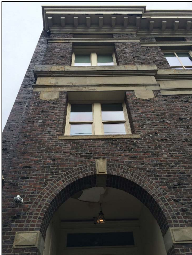
Figure 54. Below, detail view above of the club entry near the west end on the south facade.
