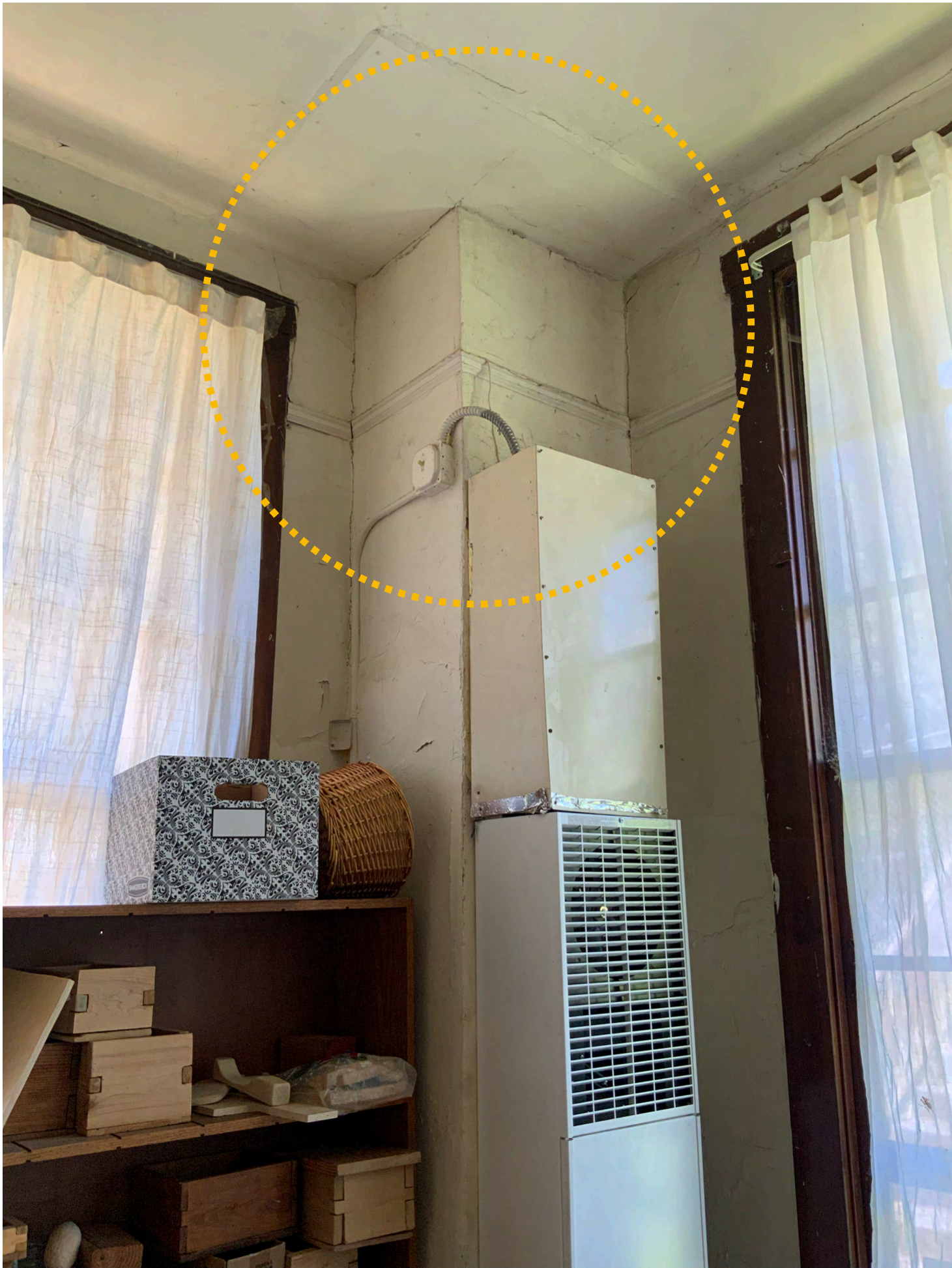
Sign of previous patches and water intrusion
