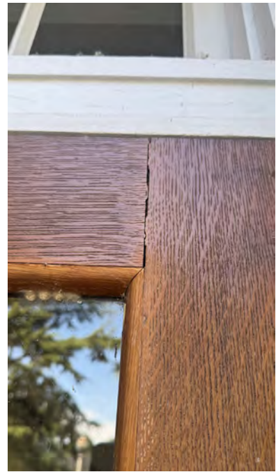
Fig. 64: Detail of gap from differential shrinkage at joint.
