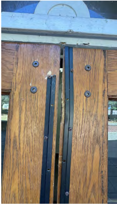
Fig. 15: Damaged astragal from forced entry.
