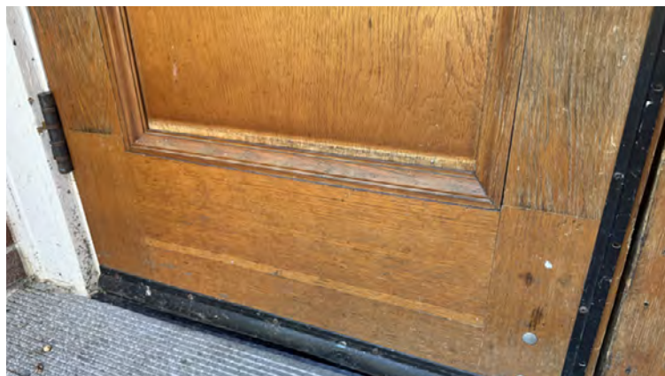
Fig. 07: Left panel of door pair S-ST04-01 shows previous rail and stile patches.
