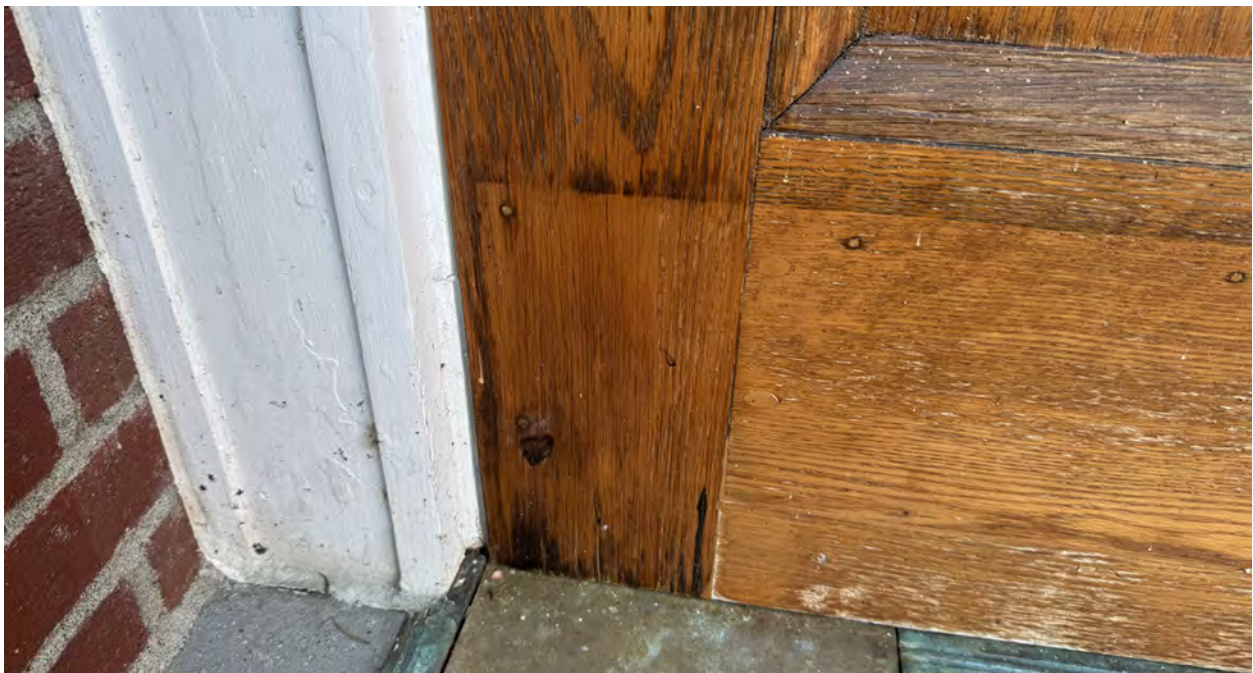
Fig. 46: Evidence of previous rot at base of door.
