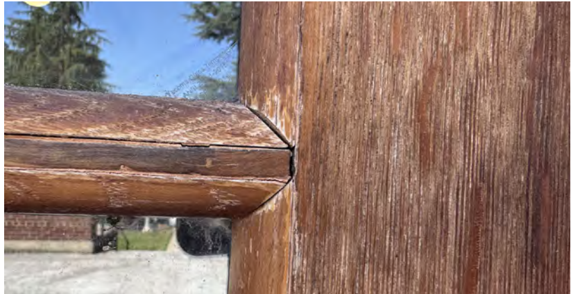
Fig. 86: Separation at joints from differential swelling.
