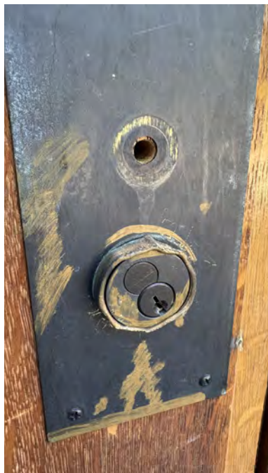
Fig. 66: Detail of damage to locks in effort to gain entry.
