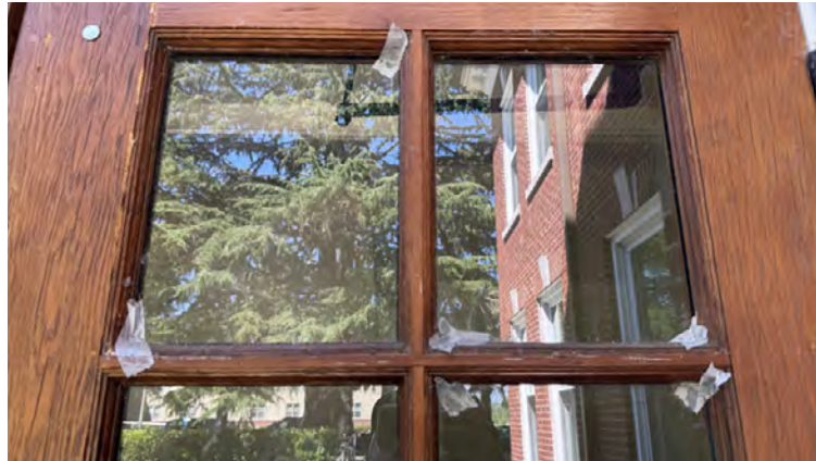
Fig. 04: Right panel of door pair S-ST04-01 following recent repair of broken lights.
