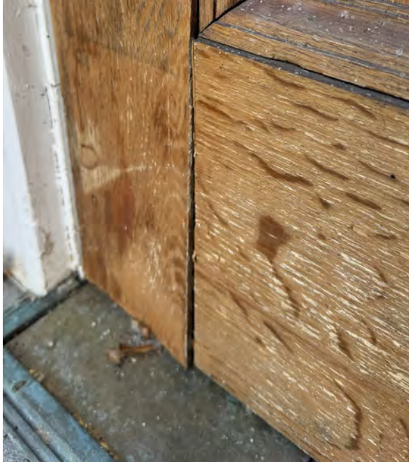
Fig. 58: Detail of misalignment due to swelling of repair wood.
