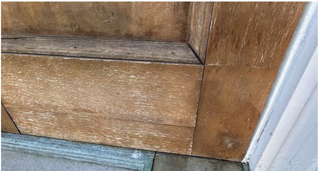
Fig. 24: Damage from moisture infiltration of failing finishes at joints causing swelling and separation of components. Details of cupping and swelling wood components.
