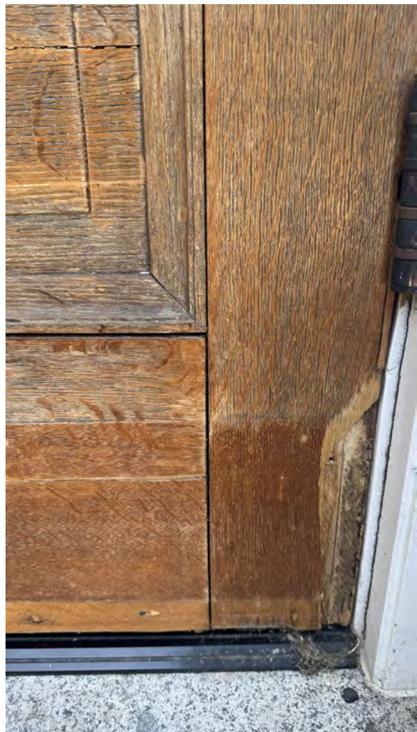
Fig. 61: Detail, loss of veneer material at base of door. Gaps from differential swelling.
