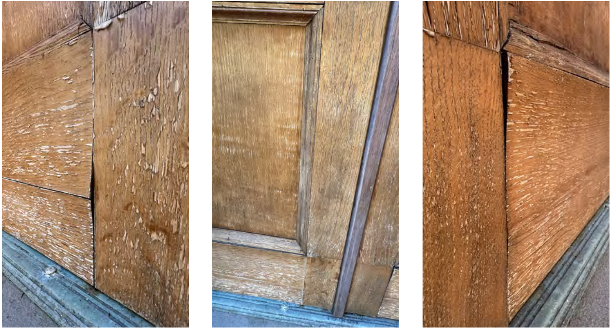
Figs. 21, 22, & 23: Damage from moisture infiltration at failing seals at joints causing swelling and separation of components. Details of cupping and swelling wood components.
