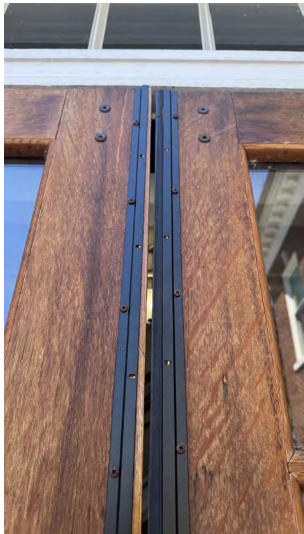
Fig. 84: Detail of door pair N-ST04-04 showing gap between doors & loss of weather stripping.
