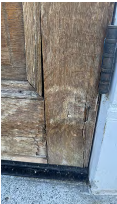
Fig. 73: Loss of veneer material from moisture intrusion.
