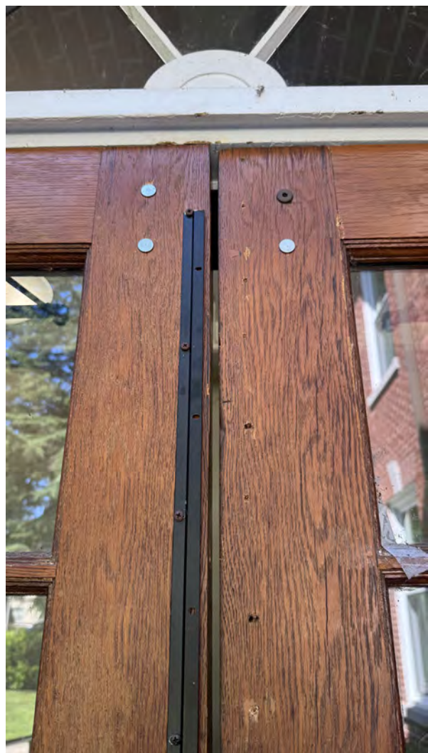
Fig. 02: Damaged and removed astragals at door pair S-ST04-01.
