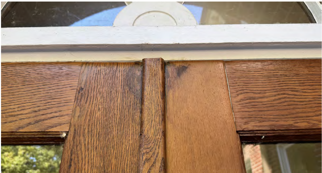
Fig. 42: Previous repair to doors visible at the rail and stile joints.
