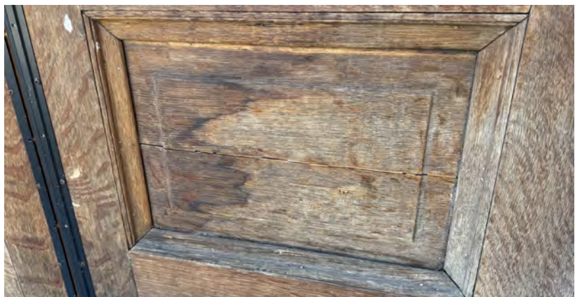
Fig. 89: Detail of cracked panel of right-hand door from forced entry attempts.
