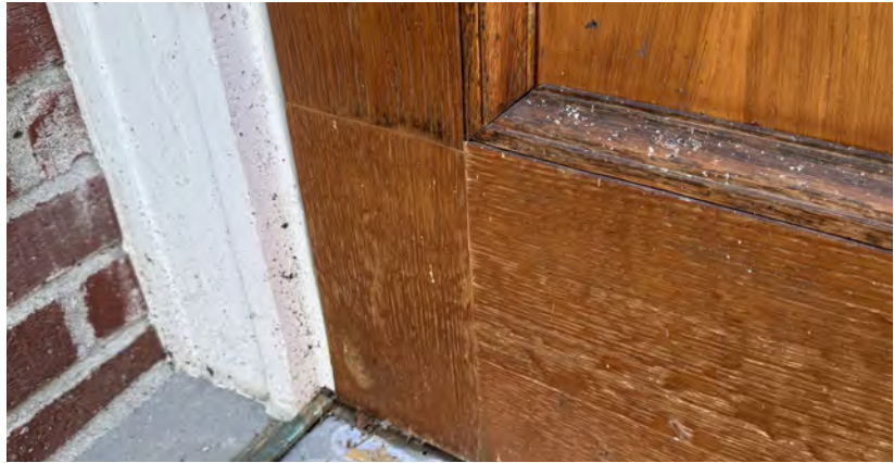
Fig. 10: Door repairs to rot during previous rehabilitation.
