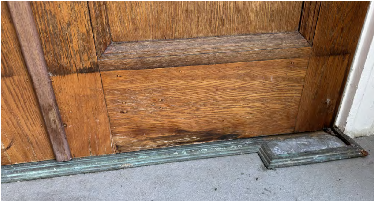
Fig. 45: Evidence of previous rot at base of door.
