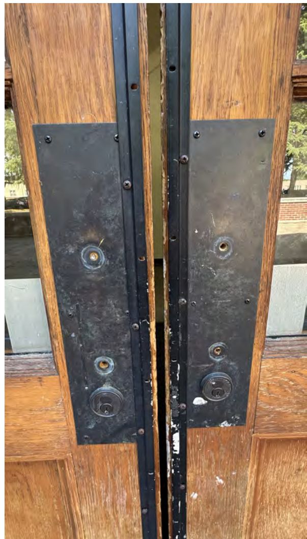
Fig. 14: Detail of damage from forced entry at doors S-ST03-06
