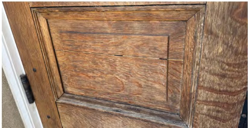
Fig. 87: Detail of cracked panel of left-hand door from forced entry attempts.
