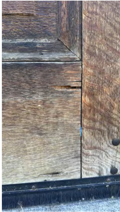
Fig. 78: Open joints from differential swelling & drying..
