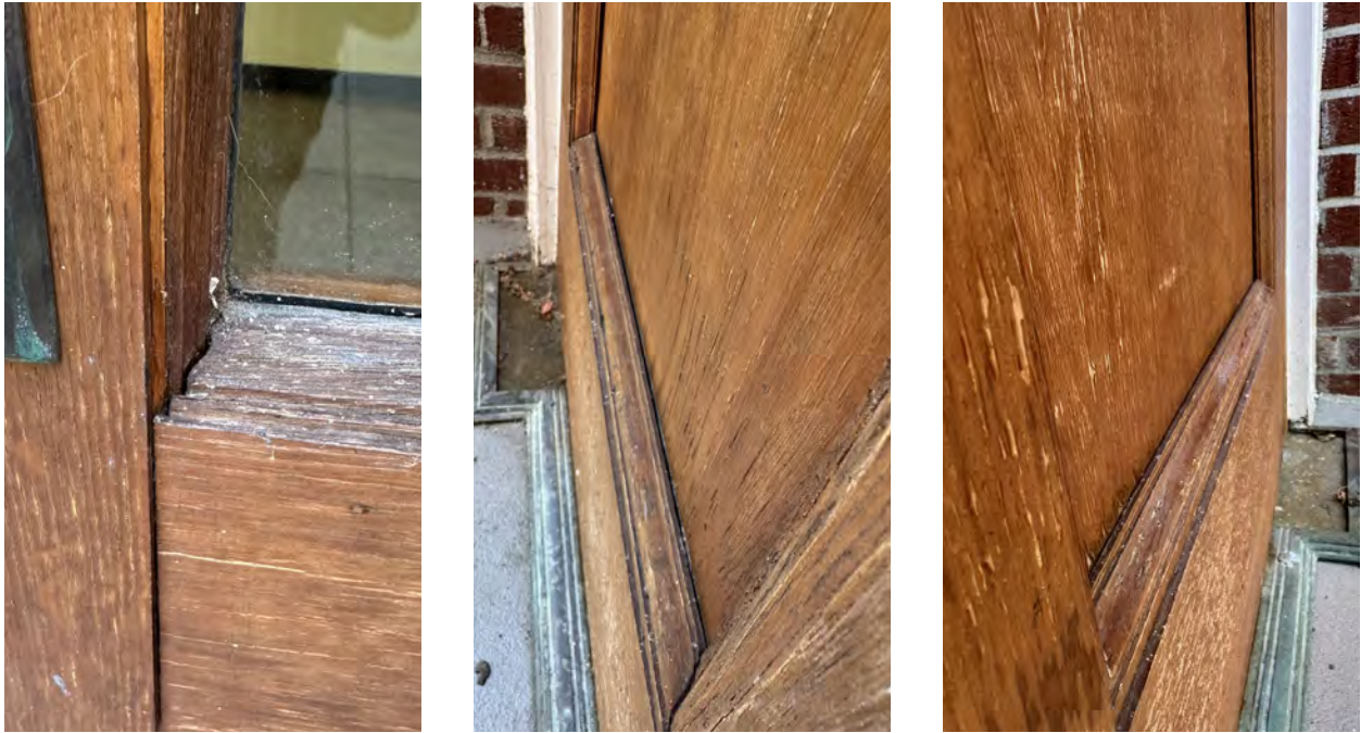
Figs. 39, 40, and 41: Details showing points of moisture infiltration from failing finishes at joints causing swelling and separation of components.
