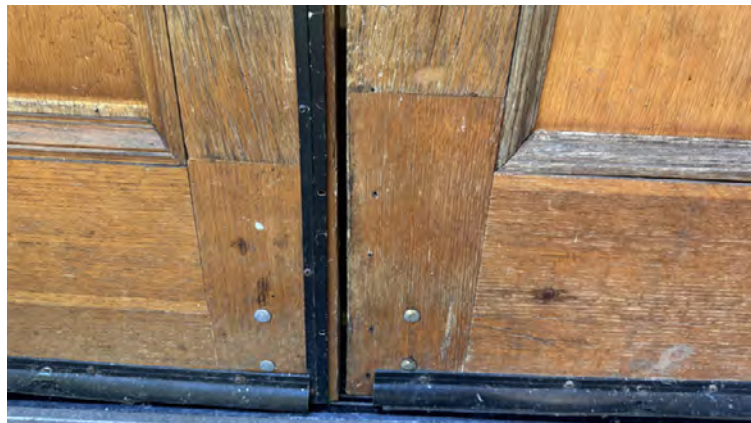
Fig. 05: Door pair S-ST04-01 shows previous rail and stile patches, and removal of astragal.
