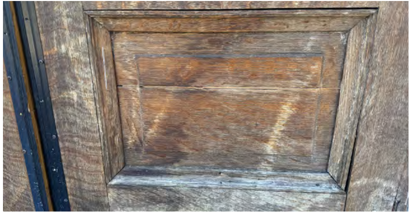
Fig. 71: Detail, exterior view of cracked panel of right-hand leaf from brute force entry attempts.
