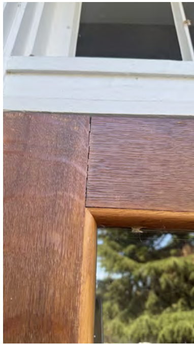
Fig. 63: Detail of gap from differential shrinkage at joint.
