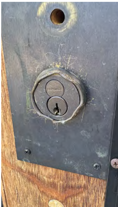
Fig. 88: Detail of damage to locks.
