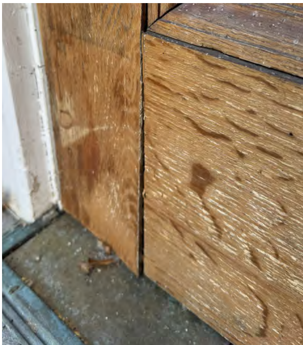
Fig. 58: Detail of misalignment due to swelling of repair wood.
