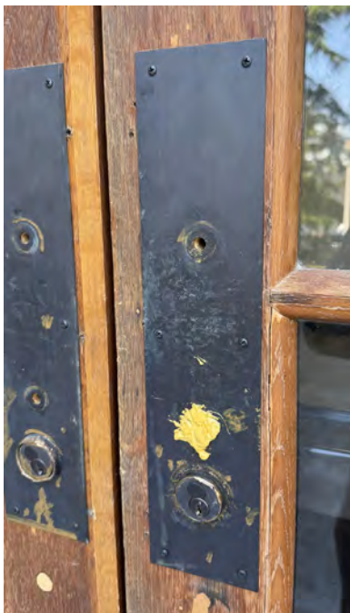
Fig. 65: Damage to locks in effort to gain entry.
