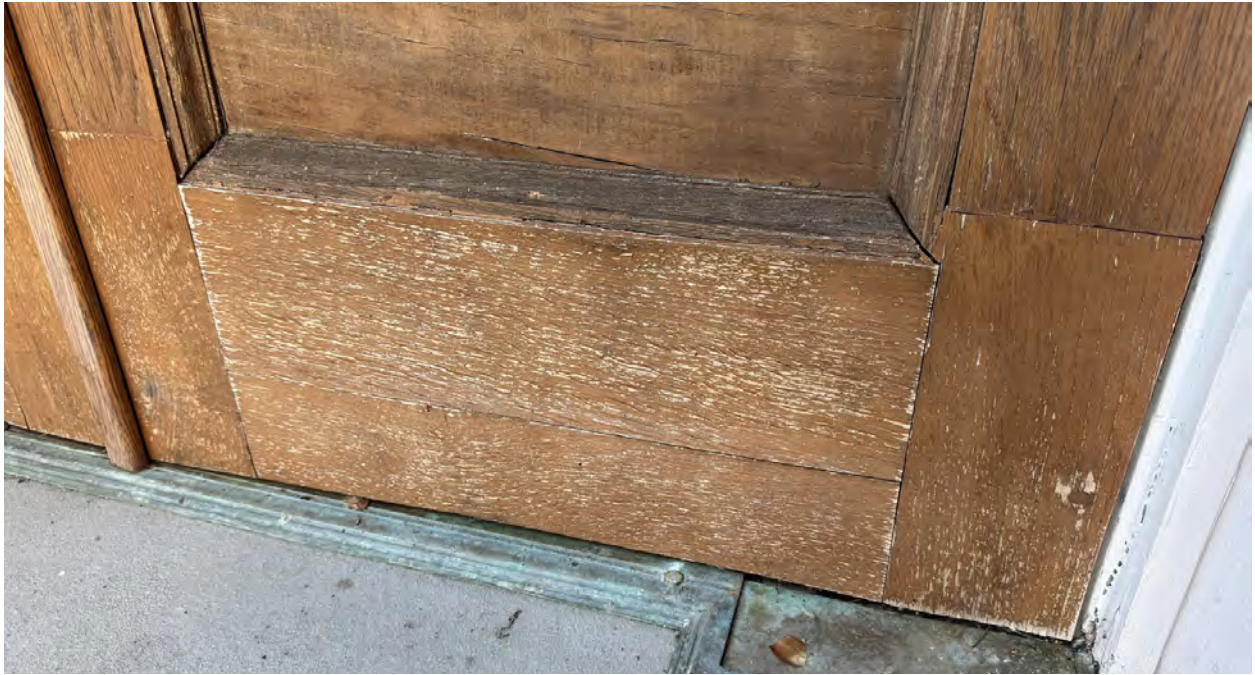
Fig. 57: Previous repairs showing gaps and butt joints misaligning created by differential shrinking.
