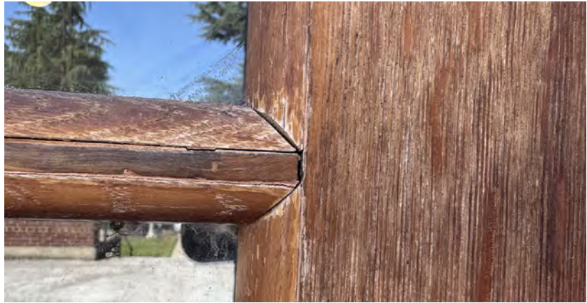
Fig. 86: Separation at joints from differential swelling.
