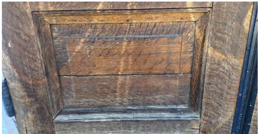
Fig. 72: Detail, exterior view of cracked panel of left-hand leaf from brute force entry attempts.
