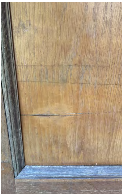
Fig. 06: Damaged panel from forced entry efforts.
