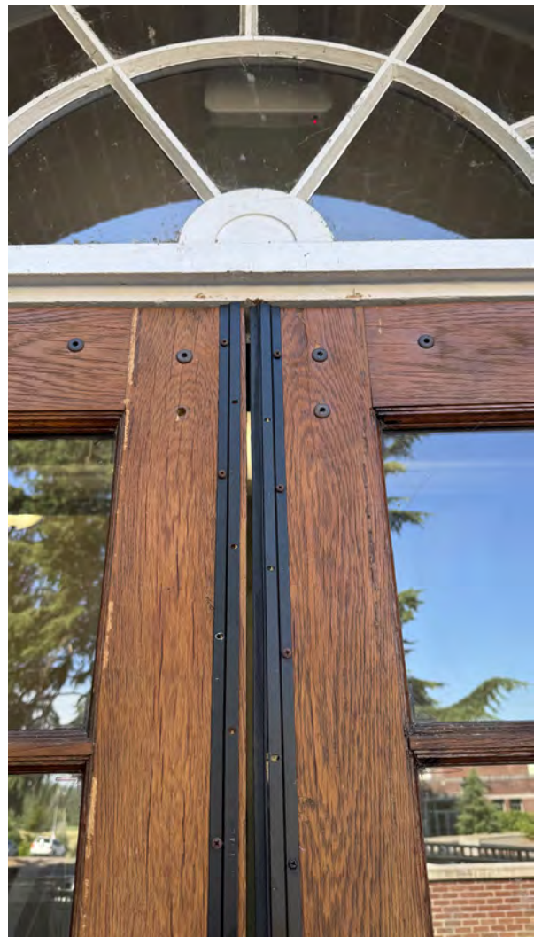
Fig. 48: Detail of door pair S-ST01-05 showing gap between leaves.
