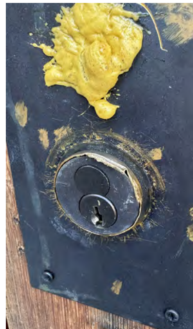
Fig. 67: Detail of damage to locks in effort to gain entry.
