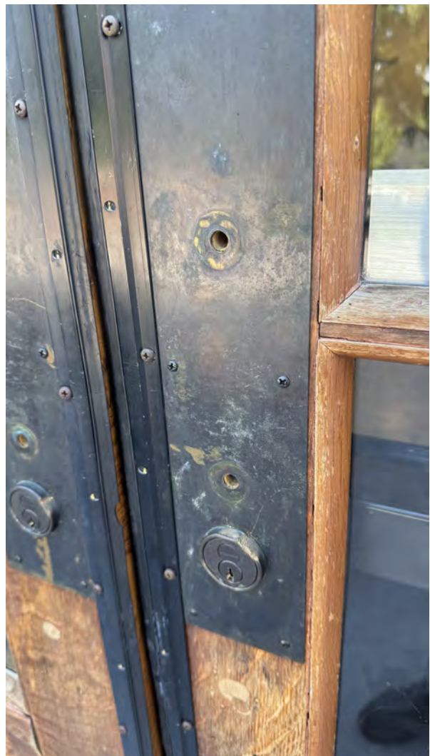
Fig. 76: Damage to door lock hardware from brute force entry efforts.
