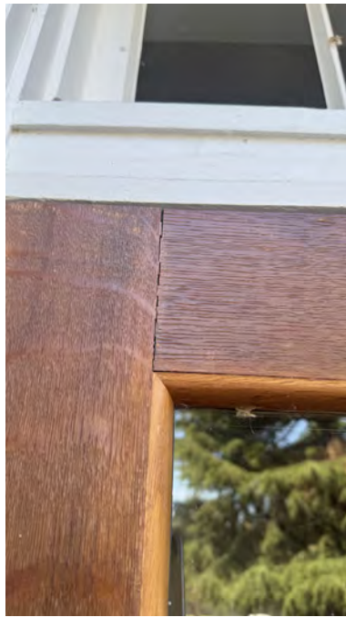
Fig. 63: Detail of gap from differential shrinkage at joint.
