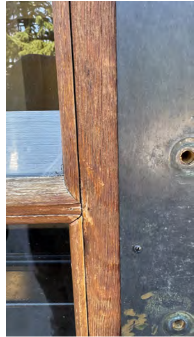
Fig. 79: Open joints from differential swelling & drying..
