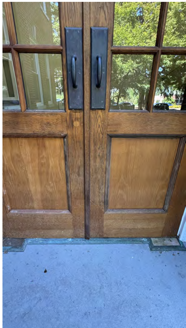
Fig. 26: Detail of doors S-ST02-05. Showing patch and repair from previous water damage.
