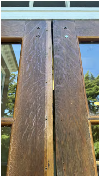
Fig. 62: Gap at door meeting. Astragals stripped from door.
