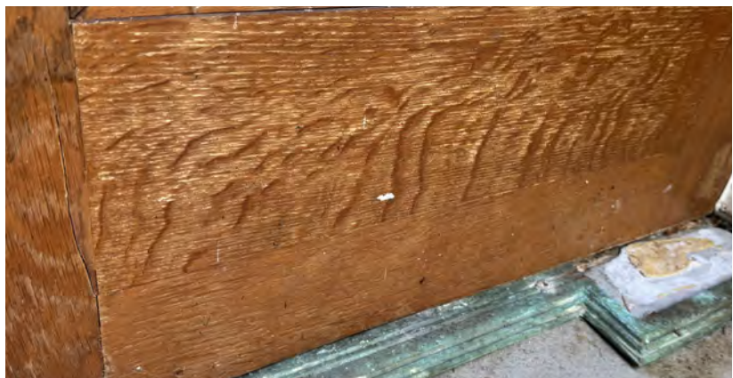
Fig. 12: Door repairs to rot during previous rehabilitation. Check in wood veneer. A crack in the stile veneer is present.
