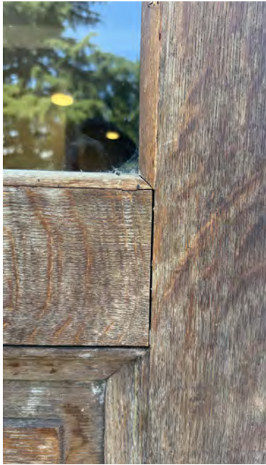
Fig. 70: Joint separation gap from differential swelling.
