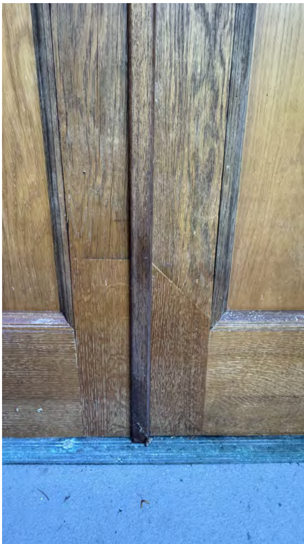
Fig. 27: Showing patch and repair from previous water damage.
