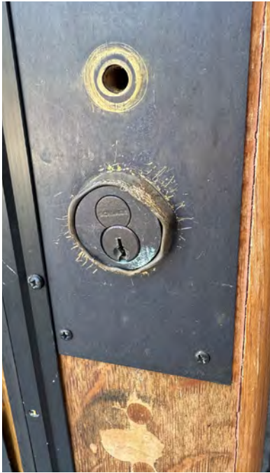
Fig. 85: Detail of damage to locks.
