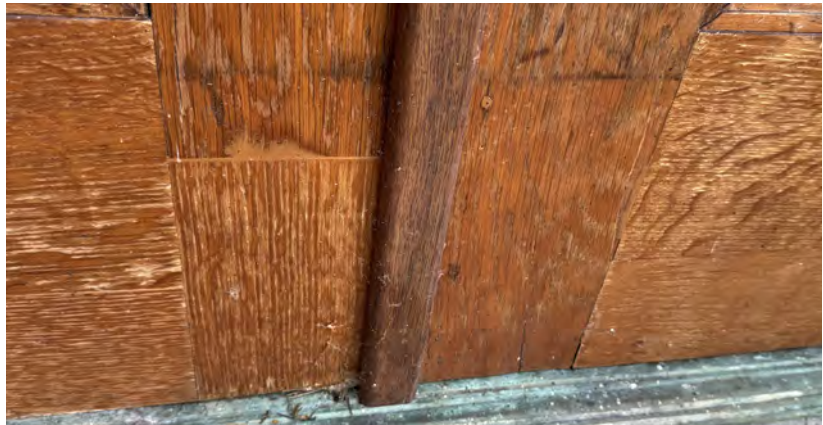
Fig. 11: Door repairs to rot during previous rehabilitation.
