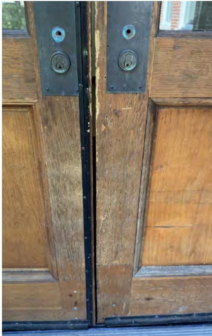
Fig. 03: Rail damage from forced entry efforts.
