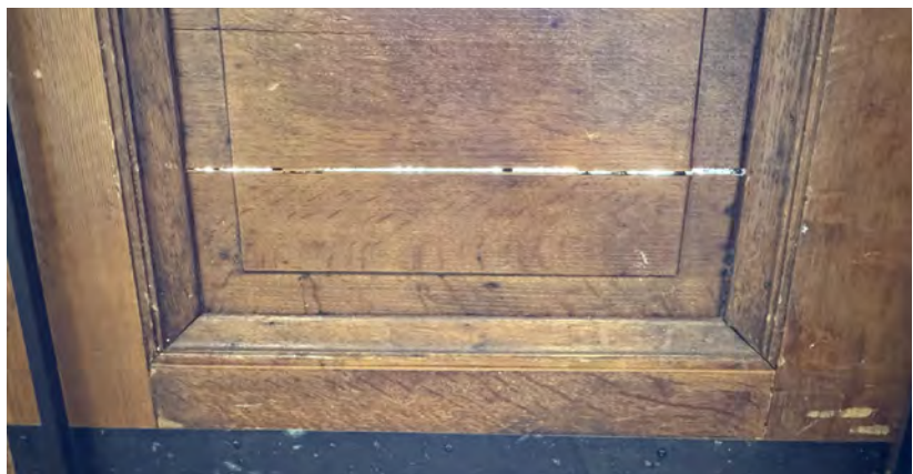
Fig. 74: Detail, interior view of cracked panel of left-hand leaf from brute force entry attempts.
