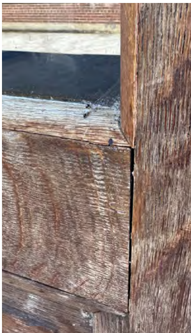
Fig. 80: Open joints from differential swelling & drying.
