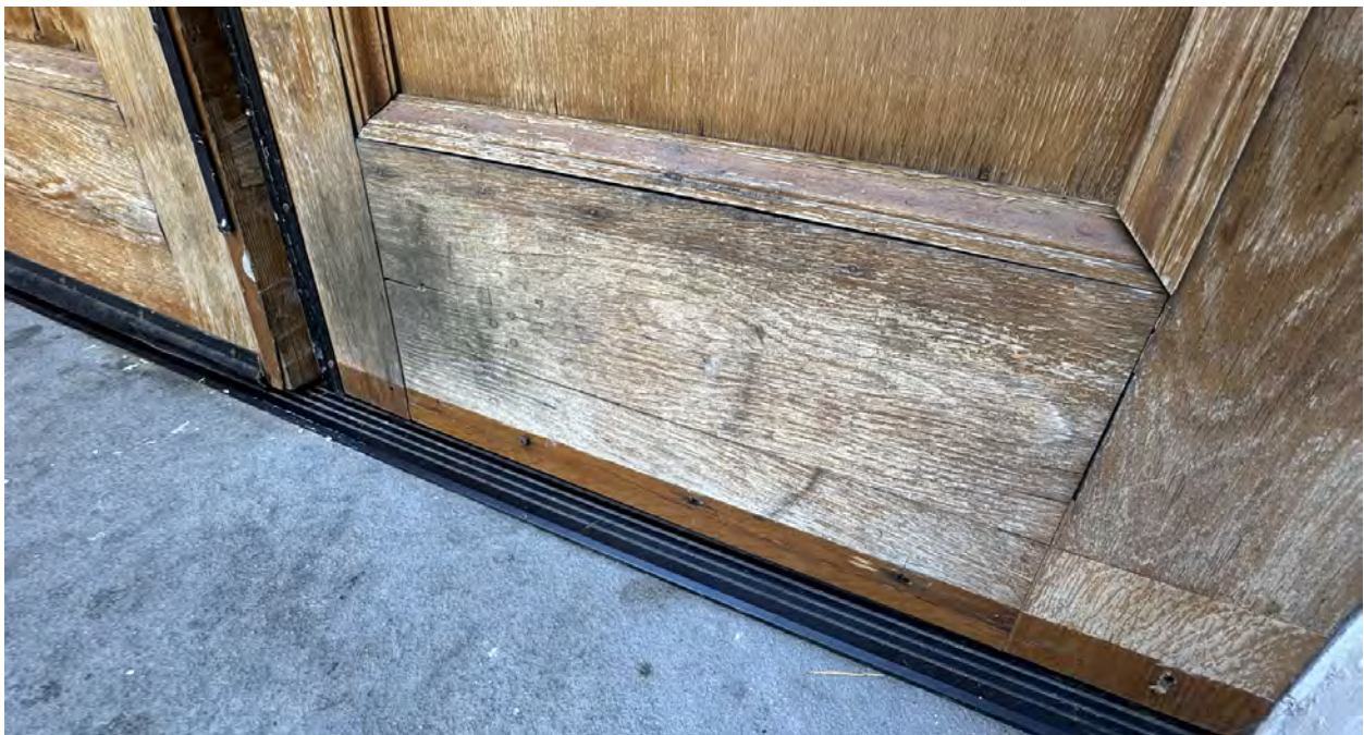
Fig. 18: Damage from moisture infiltration at failing seals at joints causing swelling and separation of components. Loss of finish due to weathering has allowed moisture to infiltrate assembly.
