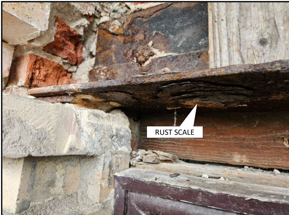
Rust scale at relieving angle.
