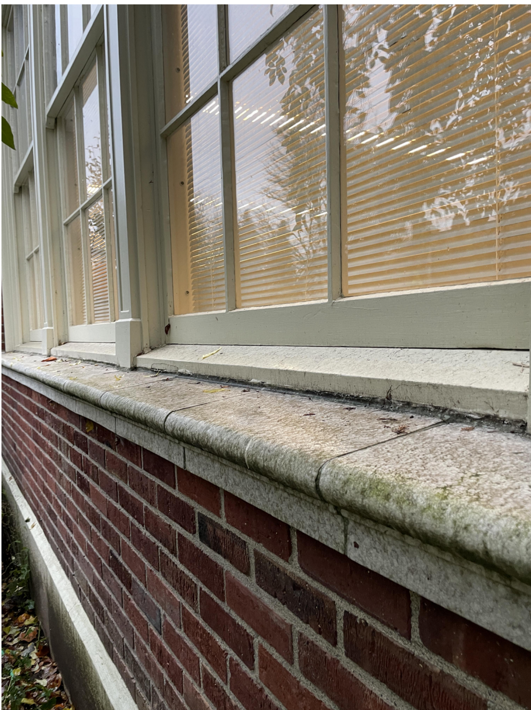
D. HISTORIC TERRACOTTA SILL
