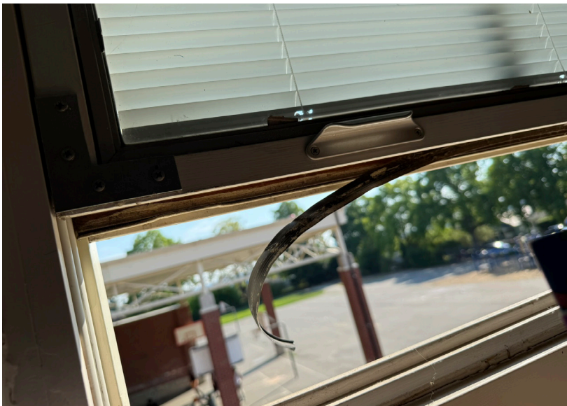
Detached or damaged weatherstripping
