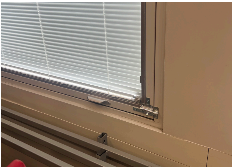
Sash hardware deterioration
