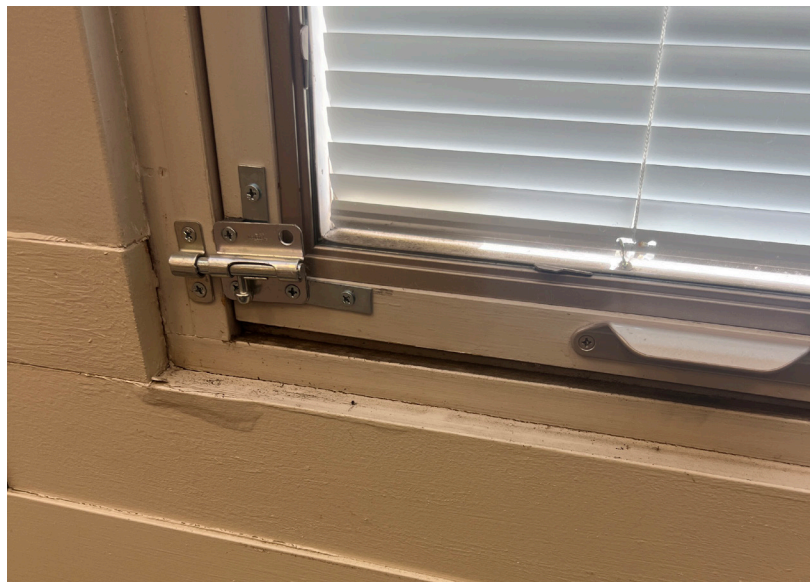
Separation between stile and bottom rail
