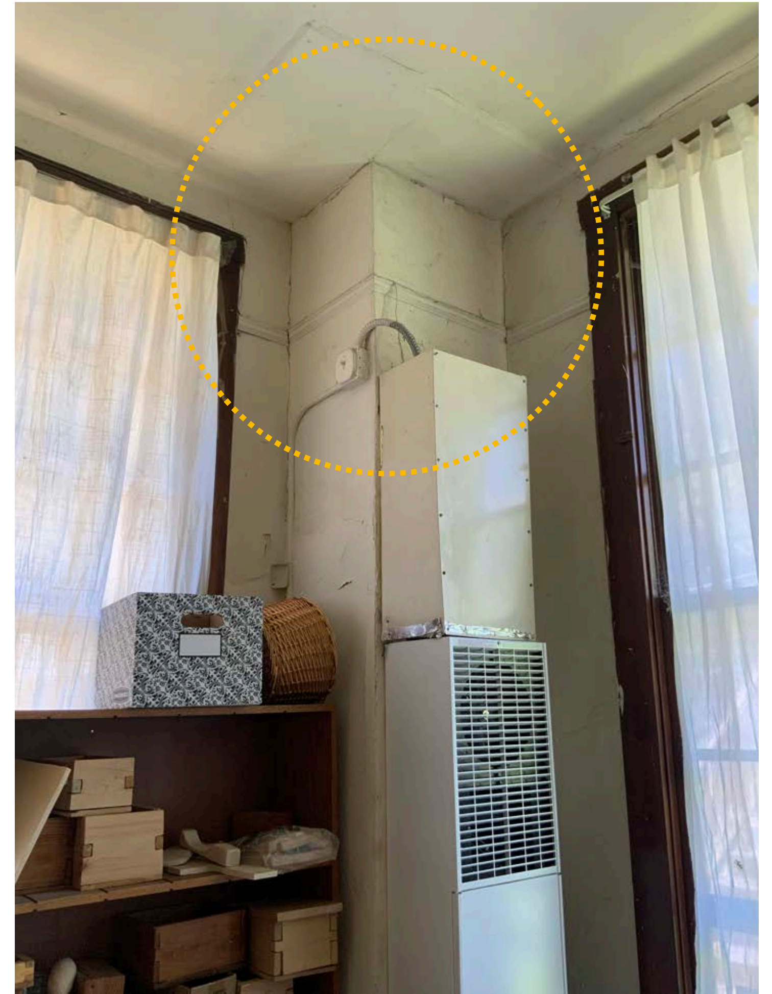
Sign of previous patches and water intrusion
