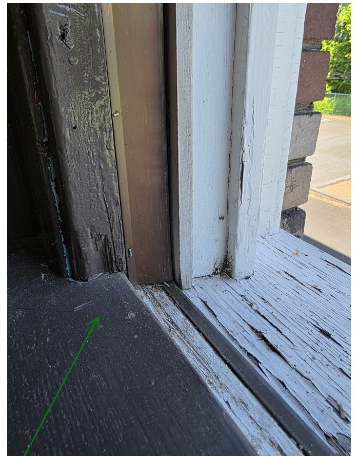
Interior case works in good condition with some chips or scratches in the paint
