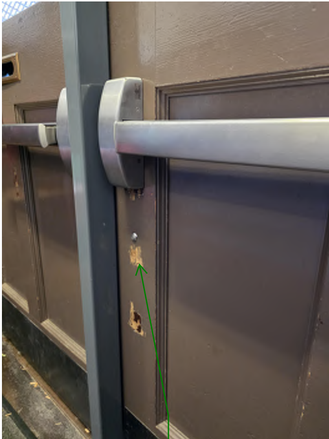
Hardware different from other doors are on main entry door. Traces of previous hardware removed remain
