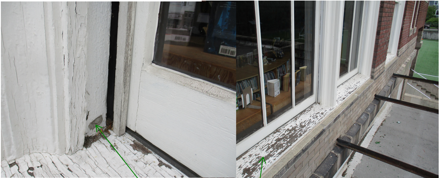
Faded paint on the exterior window sills
