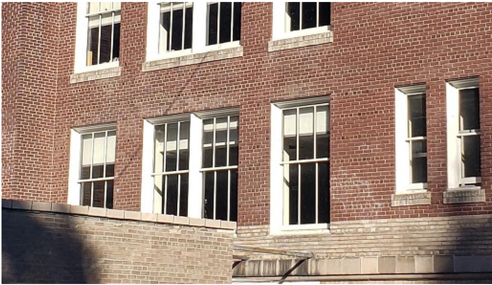
The Second floor Library window are in fair condition with minor chips in the paint observed on the jambs and some damage observed on the exterior sill due to its skyward facing nature.
