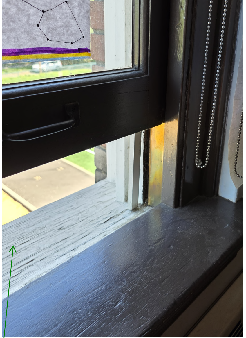
moderate weathering on exterior window sill.
