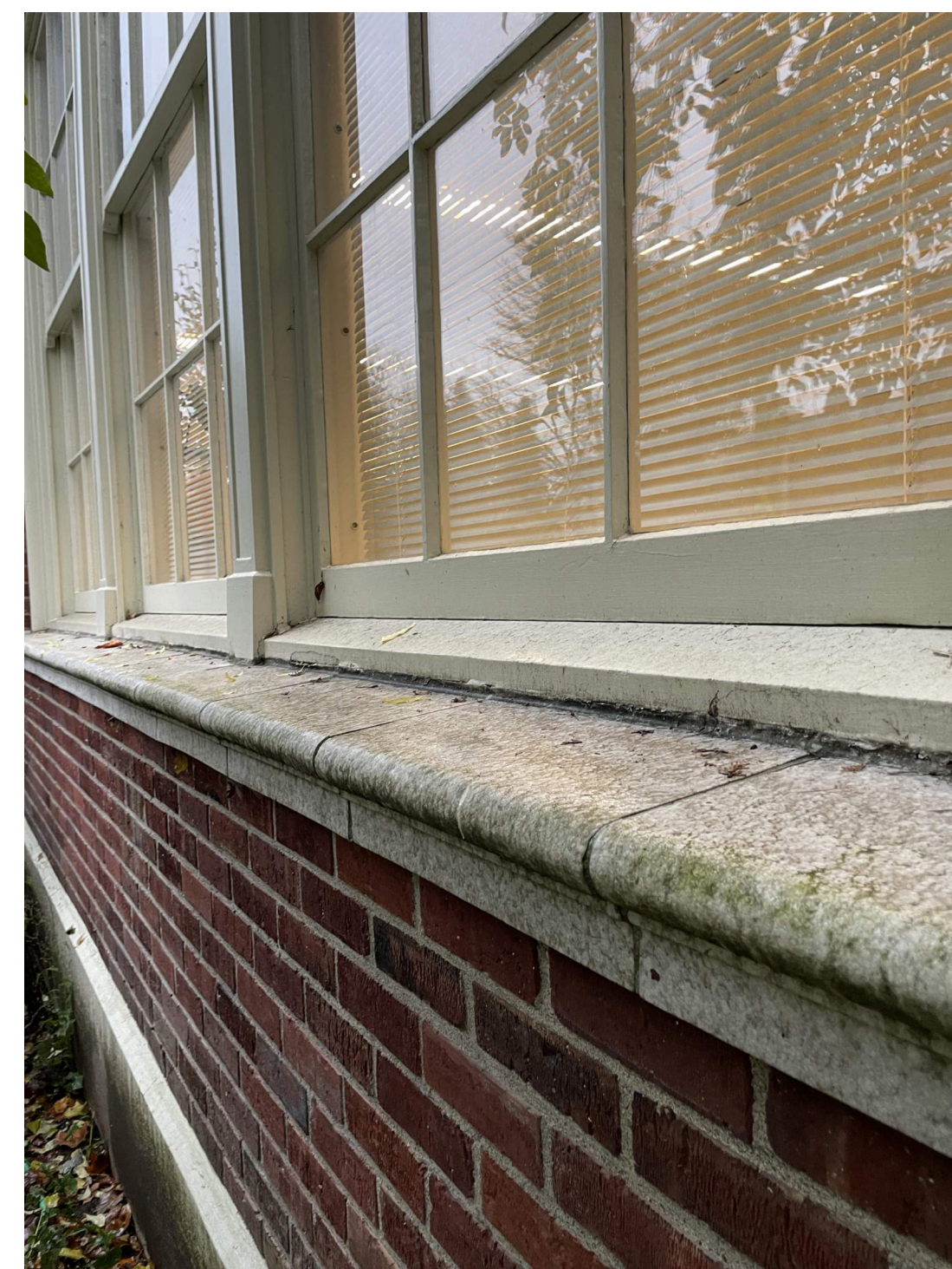
D. HISTORIC TERRACOTTA SILL
