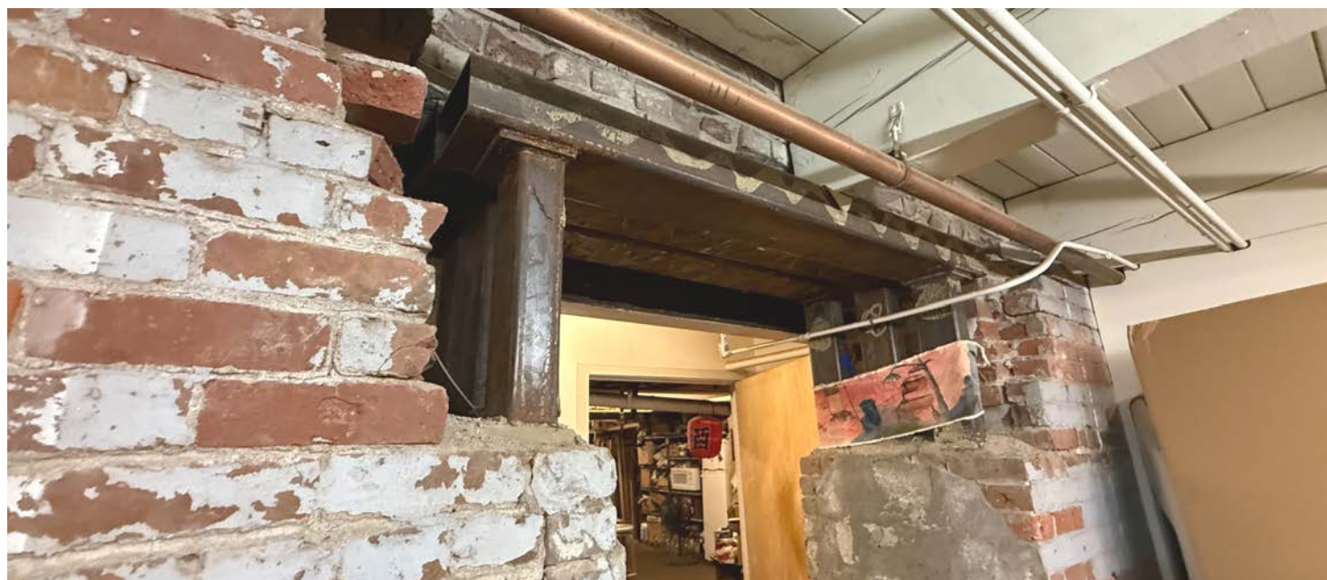
Disconnect between different portions of the building.
