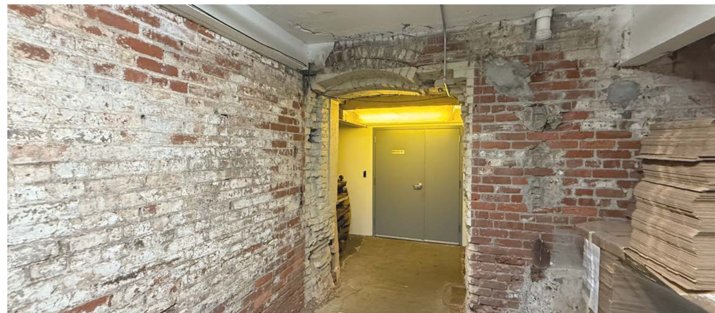
The existing configuration of the building has made strategies for providing accessibility through out the structure difficult and not cost effective.
