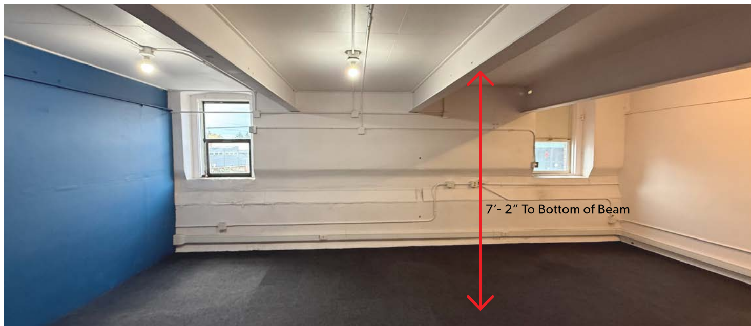
The original design for drying malts required spaces with proportions that are difficult to re-purpose into new uses, especially the original floor to floor heights
