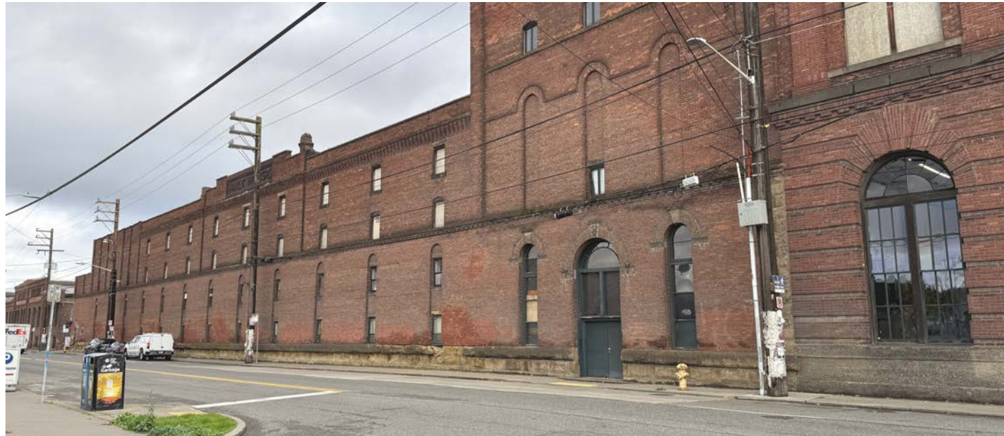
The development of Airport Way has resulted in a narrow sidewalk along the prominent west facade. This condition is further hampered by power poles and other sidewalk appurtenances
