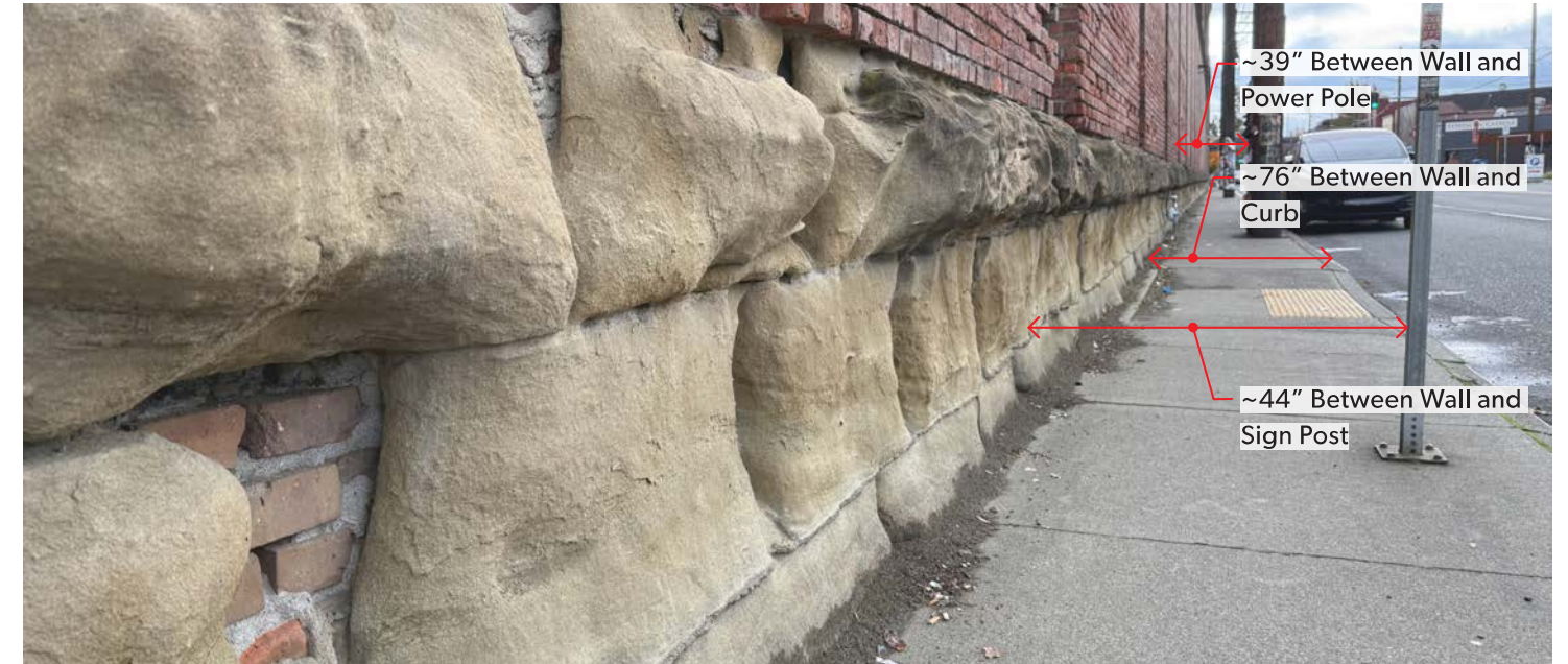
The condition of the masonry, both brick and stone, along Airport Way has significant deterioration which is assumed to be occurring due to its proximity to heavy traffic. The usability of the sidewalk is hampered by the location of the west facade in relation to the curb providing sub-optimal. The sidewalk width is further reduced by street appurtenances.
