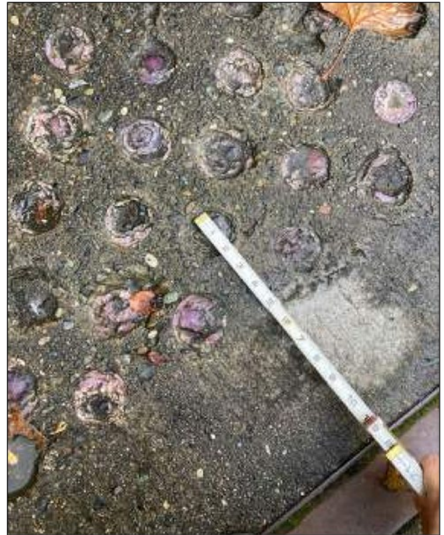
Figure 13 – Zoomed in view of the existing and deteriorated round glass pavers within the red outlined area in figure 11. The diameter is 2 inches. (Source: Seattle City Light, 2023.)
