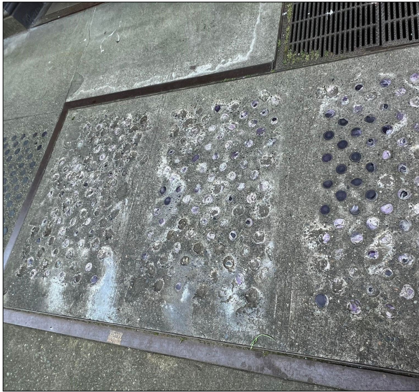
Photo 9 – Existing conditions on the exterior or sidewalk surface of the vault’s concrete hatch cover. Circular imprints are visible where glass pavers were once located in the concrete. (Source: Seattle City Light, 2022.)
