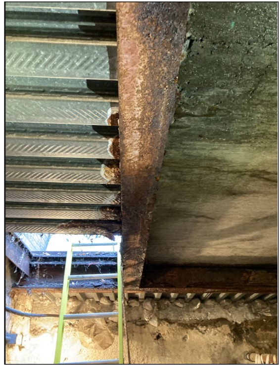
Photo 6 – Vault ceiling interior, west view showing rusted steel beams. Panel on right is sidewalk surface with glass pavers. (Source: SCL, 2022.)
