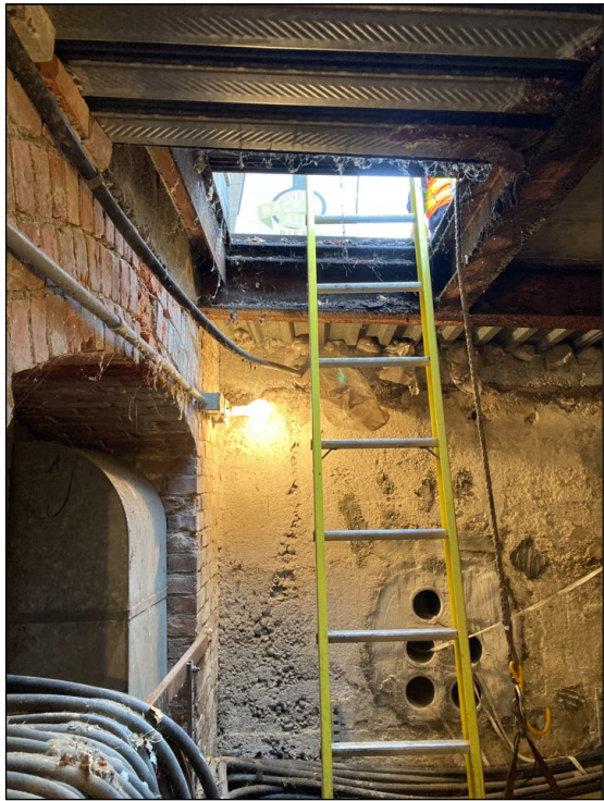
Photo 5 – Vault interior, view to the west showing existing conditions. Union Trust Annex brick arch to the left. (Source: SCL, 2022.)
