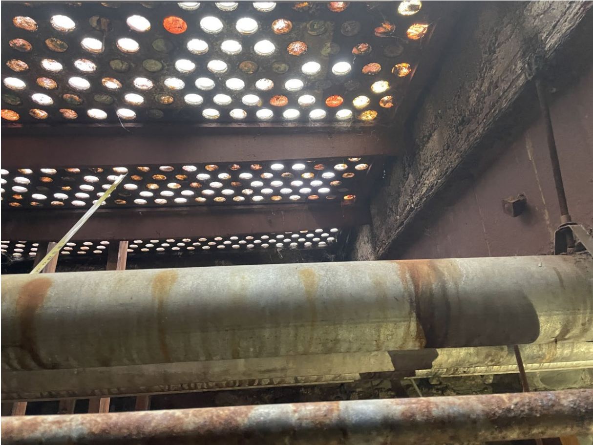
Photo 22: Underside of south frame and panel, post accident
