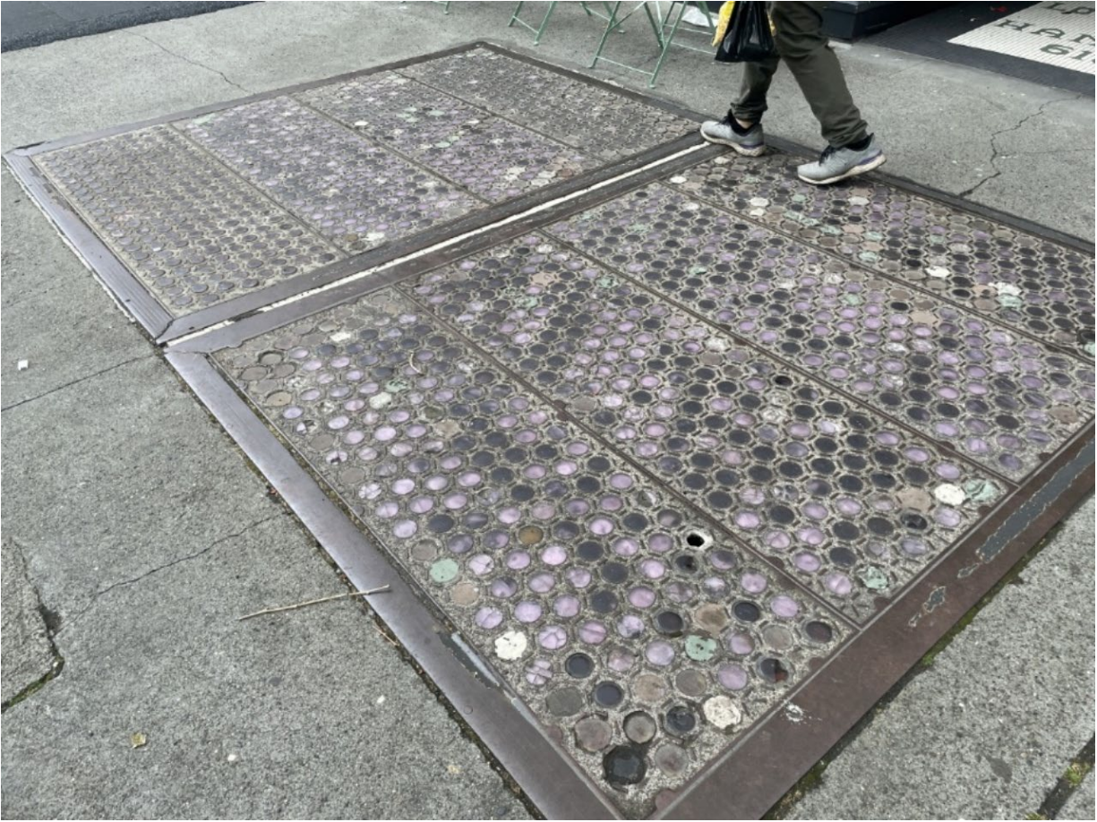
Photo 20: South frame and panel, outside, post accident condition
