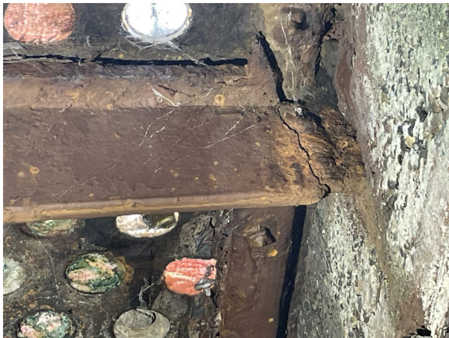
Photo 3B: Cracked cast-iron frame (typ)
