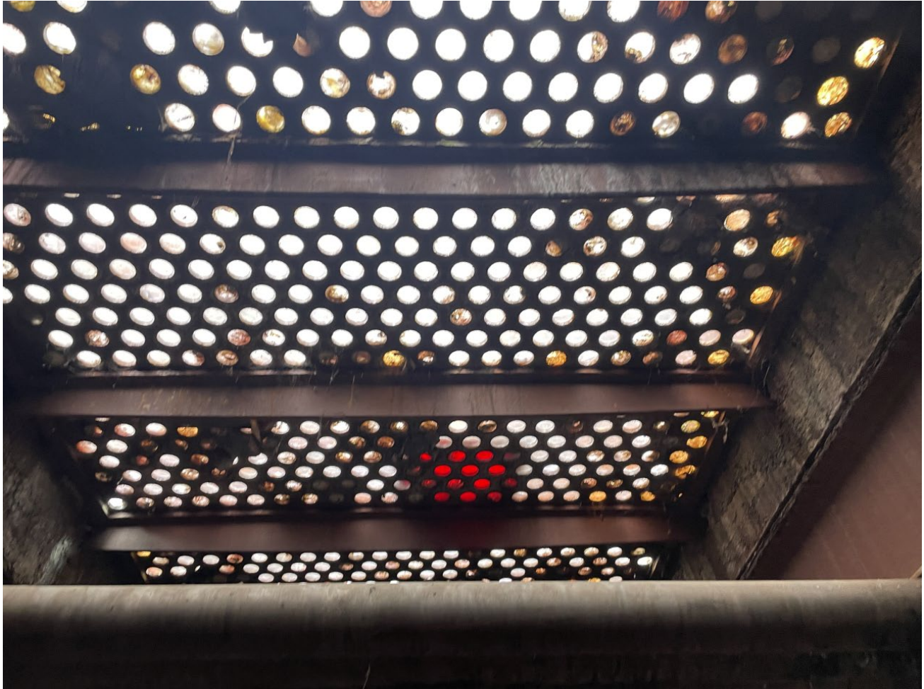
Photo 24: Underside of South frame and panel, post-accident condition
