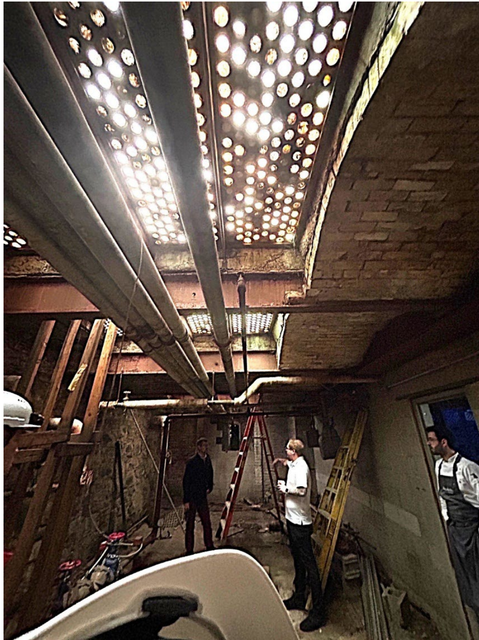
Photo 15: Looking north interior view of areaway – post accident
