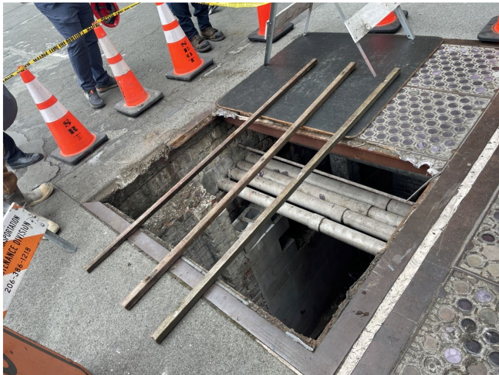
Photo 2: North frame and panel, post-accident condition
