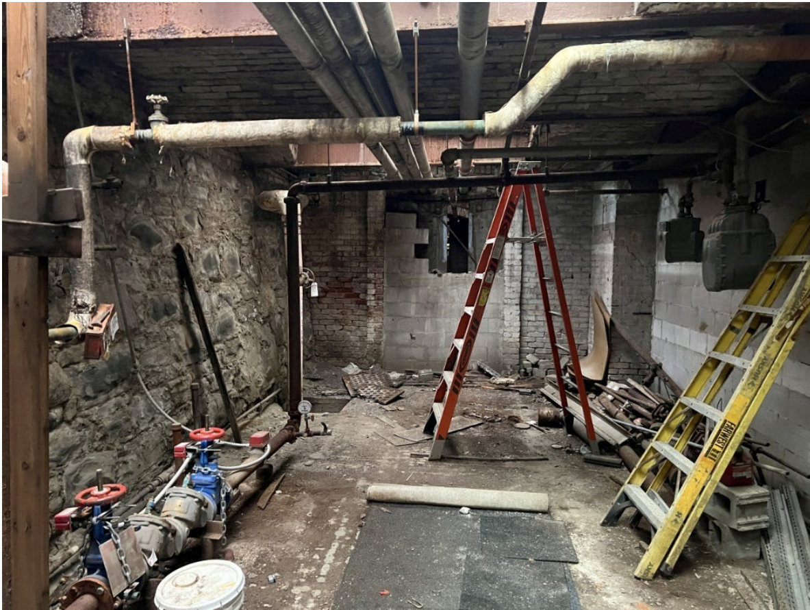
Photo 13: Looking north interior view of areaway – post accident
