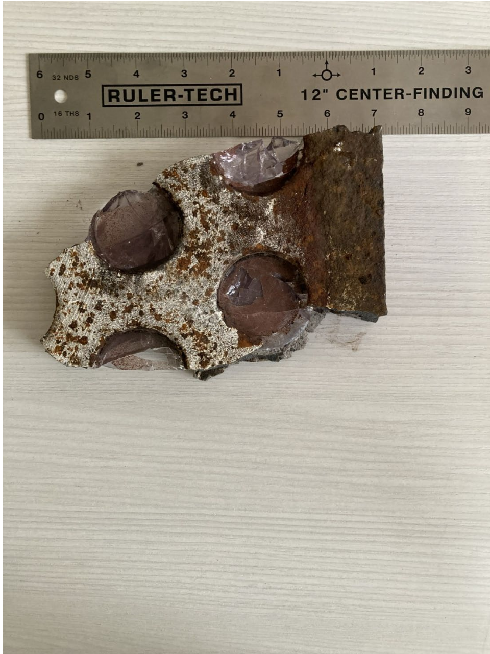
Photo 8: Underside of a fragment of cast-iron panel
