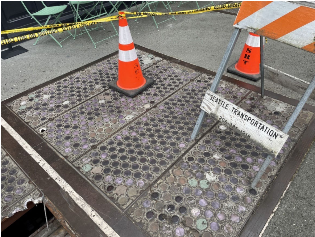
Photo 1: North frame and panel, post-accident condition
