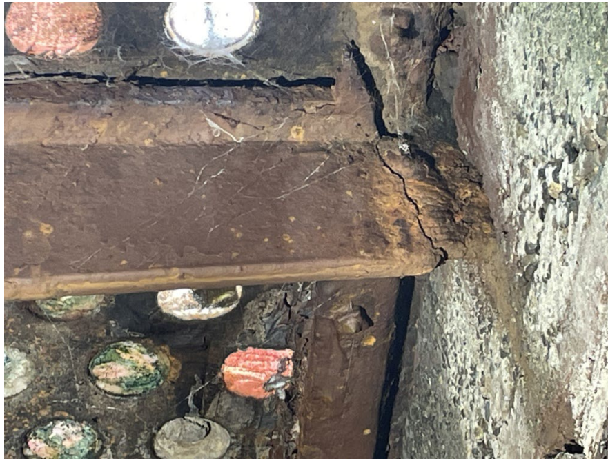
Photo 3A: Crack cast-iron frame (typ)
