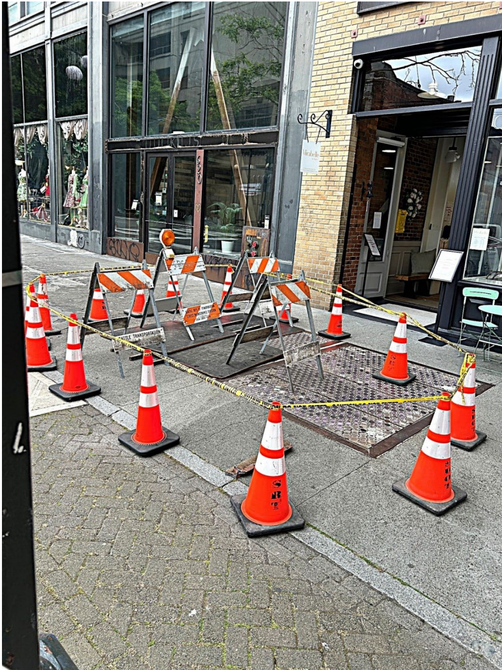
Photo 17: Post accident condition
