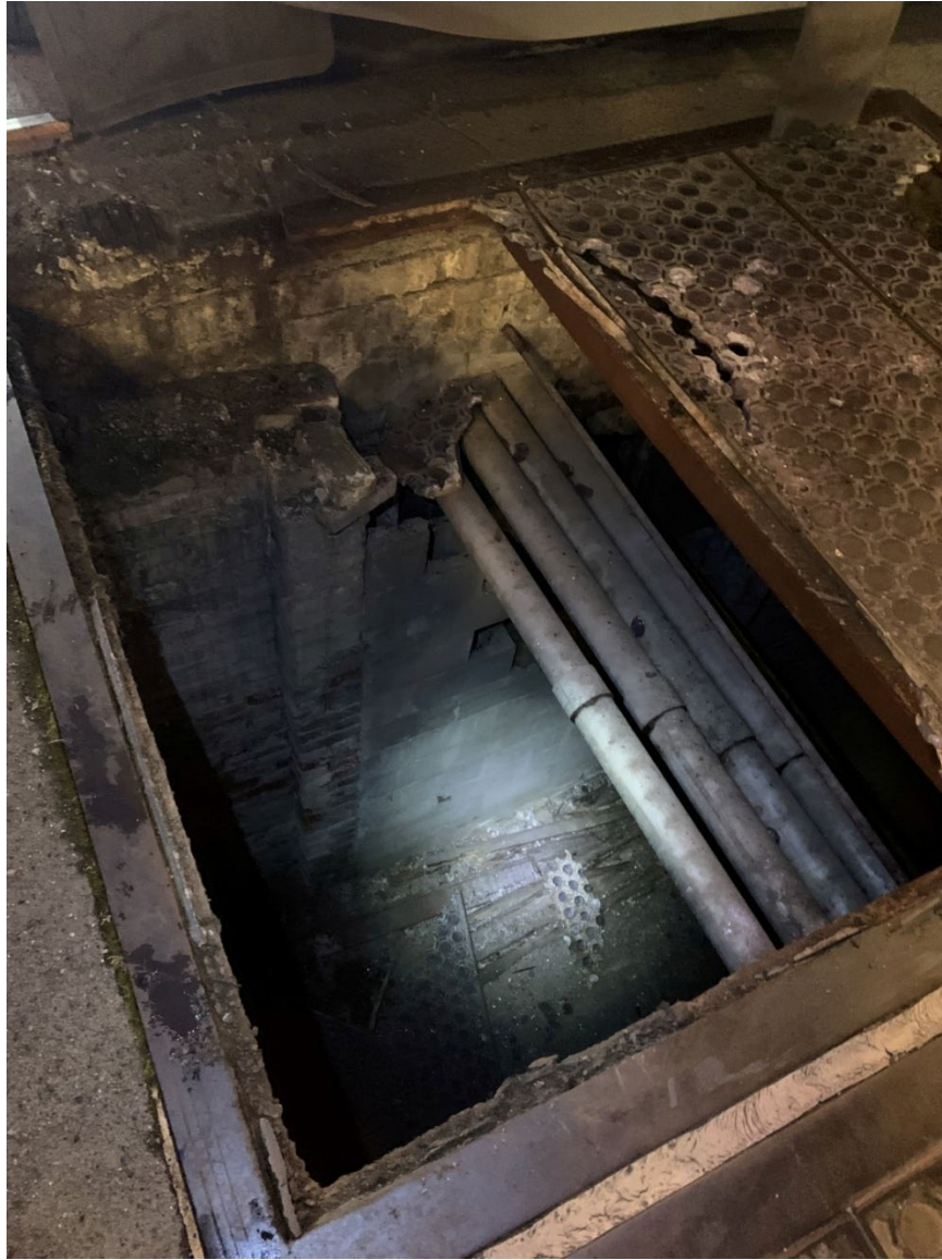
Figure 2: Damage of north skylight right after vehicle was removed lifted from the opening
