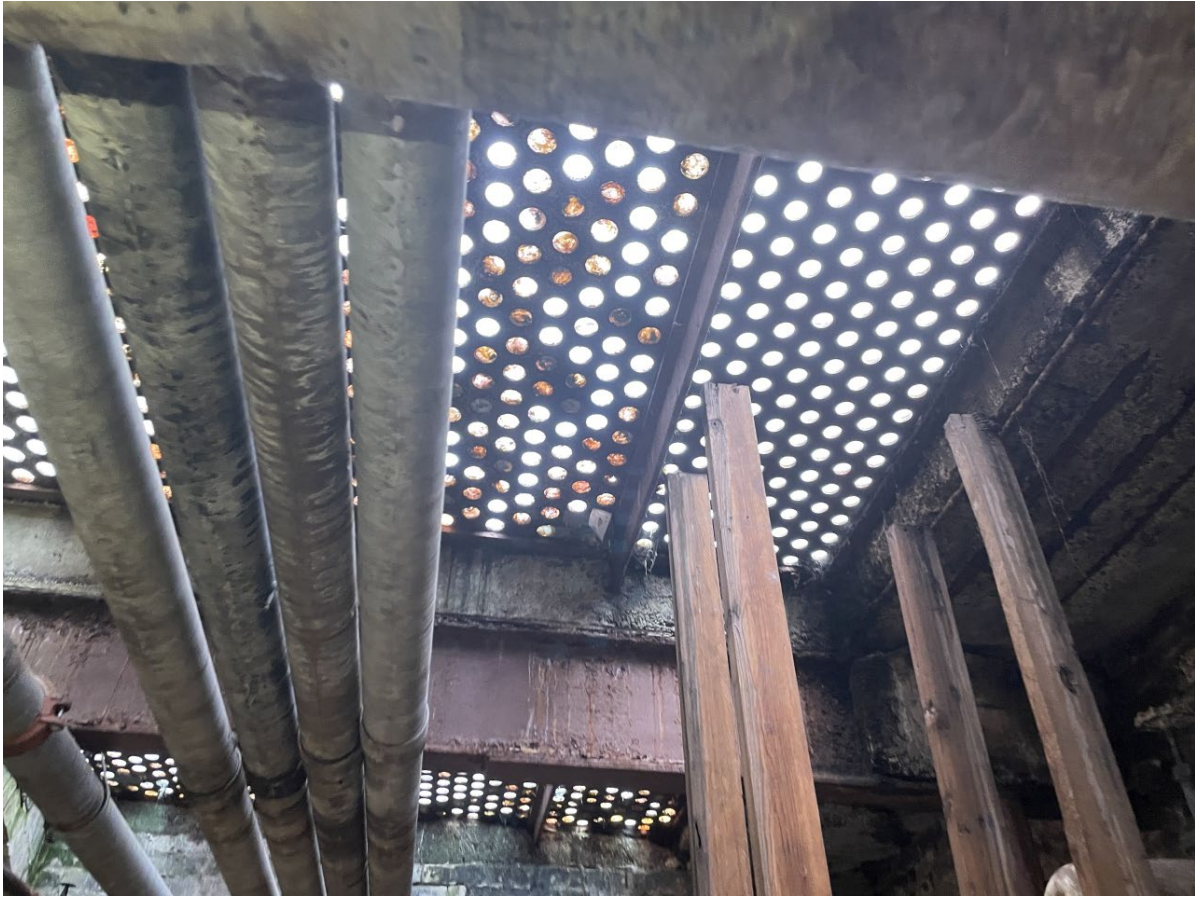
Photo 23: Underside of south frame and panel, post accident
