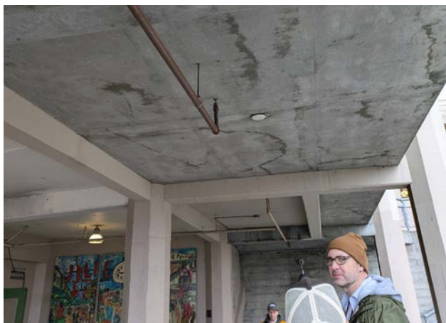
Level 3 bays with no fixtures.
