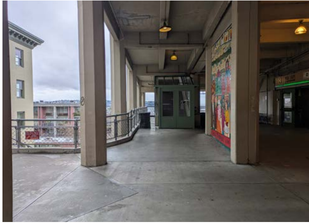
Example of existing Level 4 lighting.
