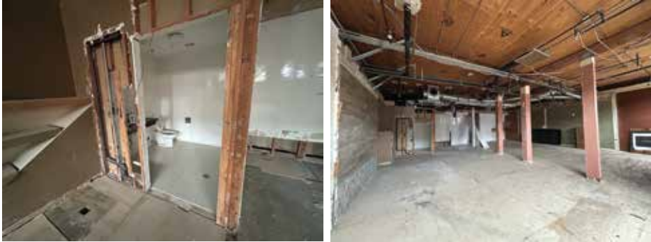
CURRENT CONDITION: Interior unfinished/unappealing at street view
