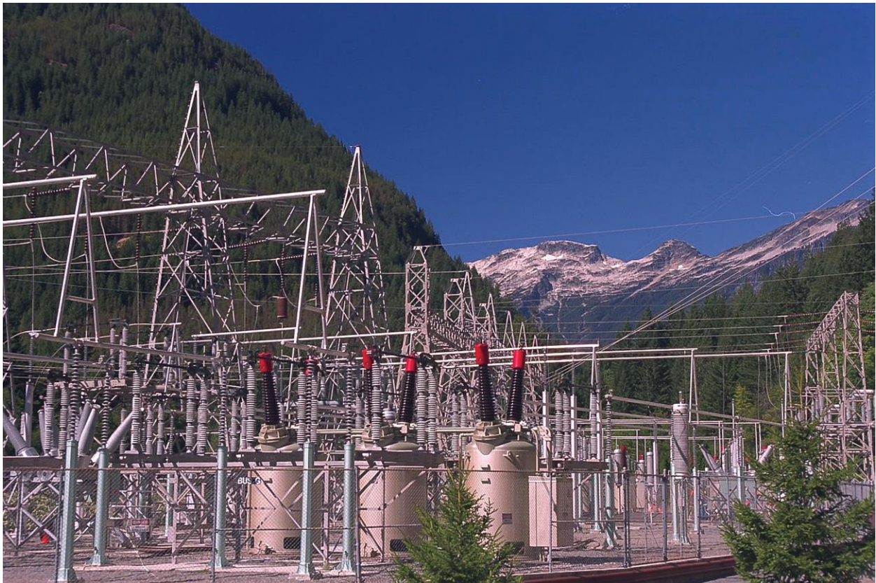
The Diablo switchyard in the North Cascades with Elephant Butte in the background.
