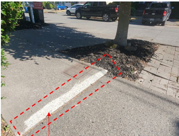
Example of a bevel : Edge of sidewalk was ground down so it matches the height of the neighboring concrete panel.
