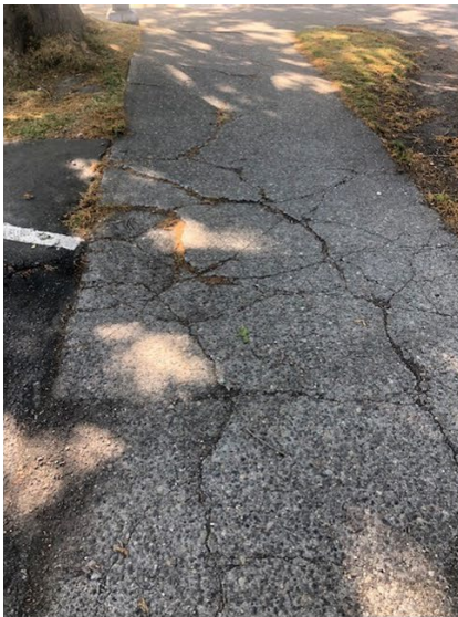
Extreme cracking on a segment of sidewalk near Lighthouse for the Blind.
