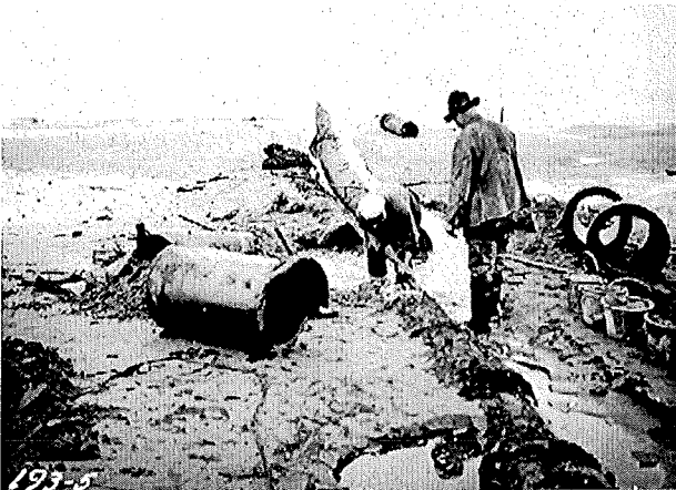
53 rd Ave. S.W. Outfall [lawing sewer pipe at low tide], Sept. 20, 1934 Dept. of Streets and Sewers Photographs, Item No. 38615
