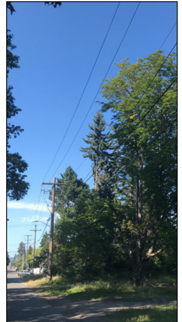
Delridge utility poles (photos: Vaughn Bell).
