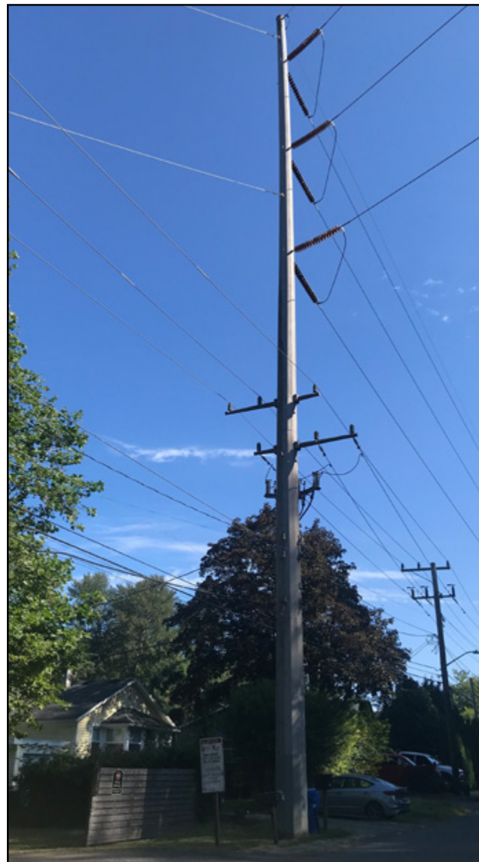
Delridge utility poles (photos: Vaughn Bell).
