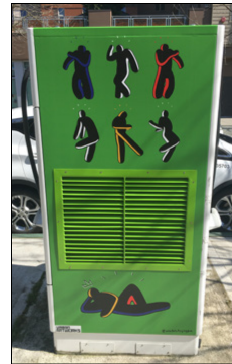
Anatol Steck, Seattle City Light Beacon Hill electric vehicle service cabinets.
