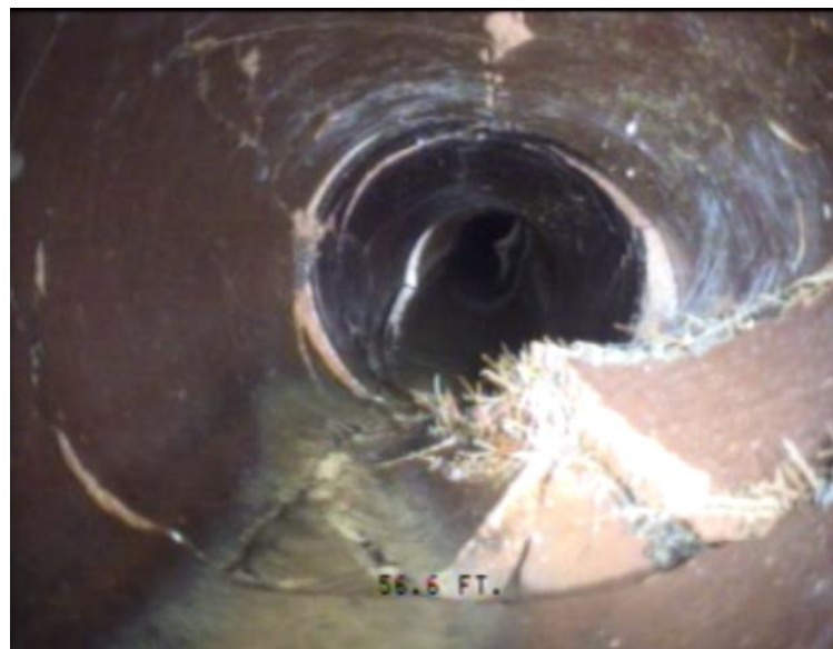
Broken Deformed – Roots
