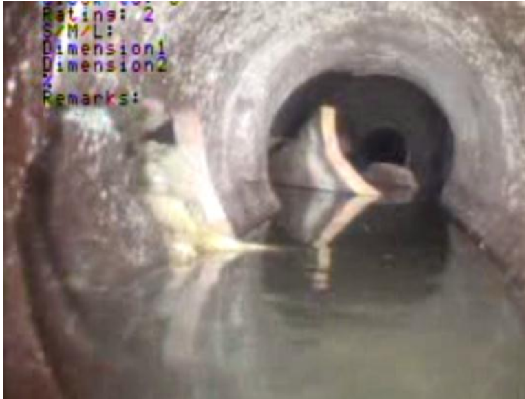
Collapse – Significant Blockage
