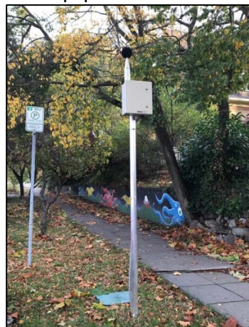
Photo 2. Equipment at Location 2
