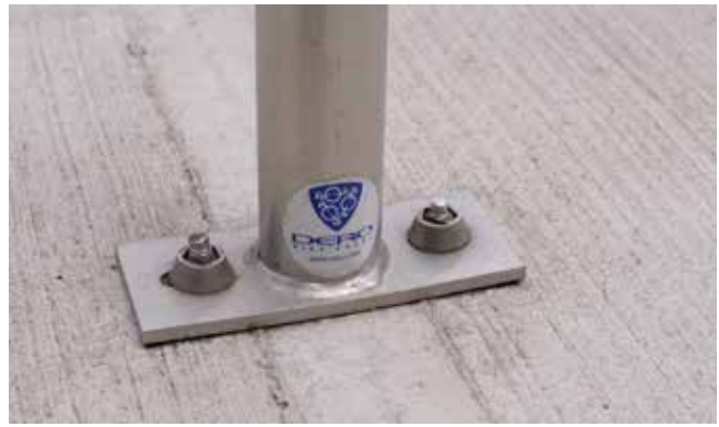
Tamper-proof hardware (Photo: MIG/SvR)
