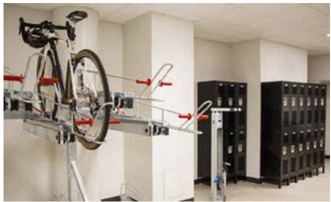
Bike room with stacked racks, service station and lockers (Photo: Dero)
