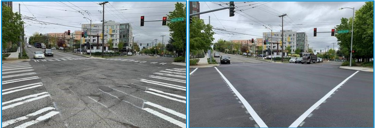
Before and after paving on 12 th Ave S and Boren Ave S. Crosswalk markings will be replaced, as well.
