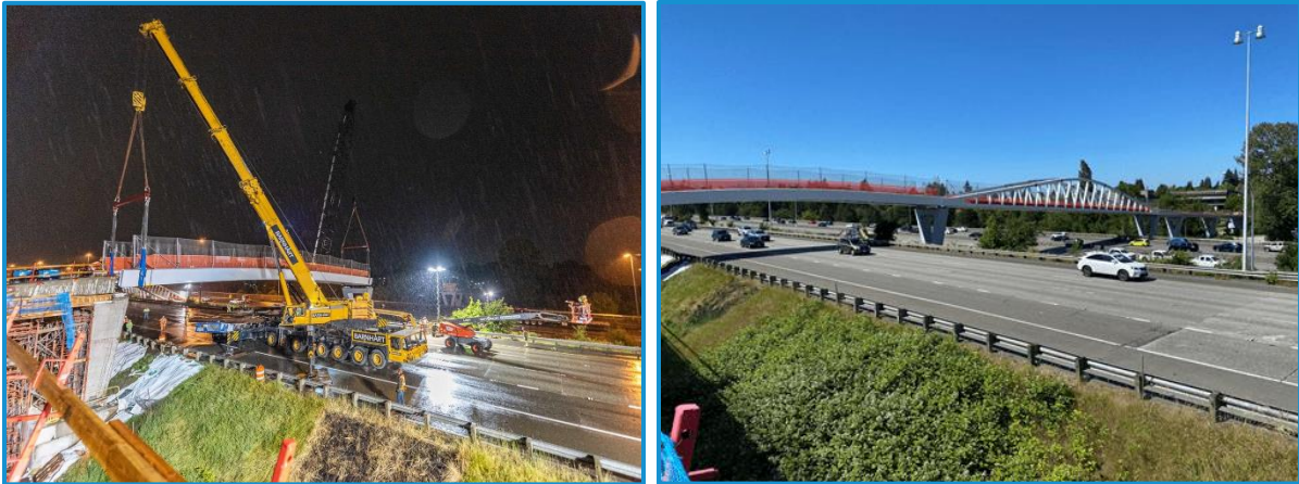
Early on June 13 and 20, the Northgate Pedestrian and Bicycle bridge spans were installed. Photo Credit: Tim Durkan.
