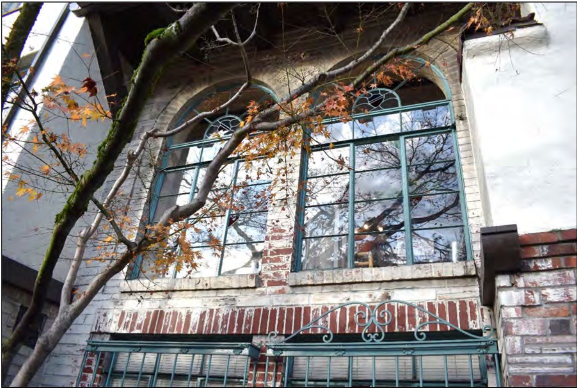
Fig. 18 - West elevation, detail of arched double window, metal window screens, masonry, stucco.
