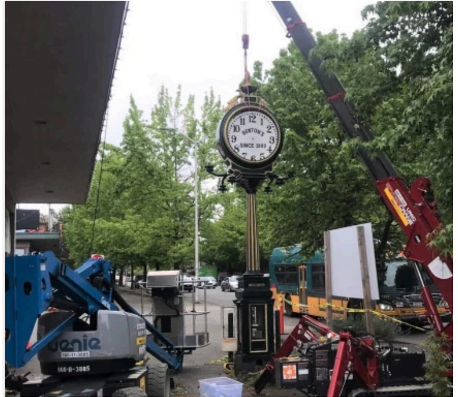
2020 - BENTON JEWELRY STREET CLOCK DURING THE MOST RECENT REMOVAL ON LAURELHURST NEIGHBORHOOD FOR FUTURE RELOCATION. THE ORIGINAL LOCATION OF THE CLOCK WAS ADJACENT TO THE ORIGINAL BENTON JEWELRY IN UNIVERSITY WAY.
