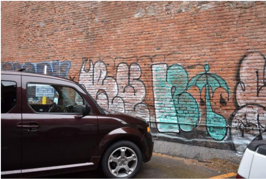
5 - Tagging on north wall continuing at the middle of building. .
