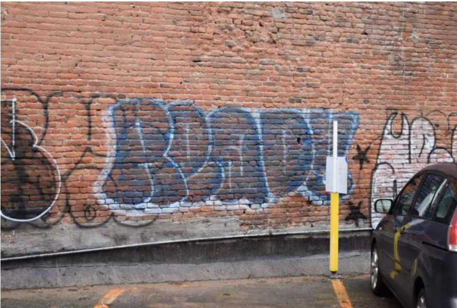
4 - Tagging on north wall near the middle of building. .
