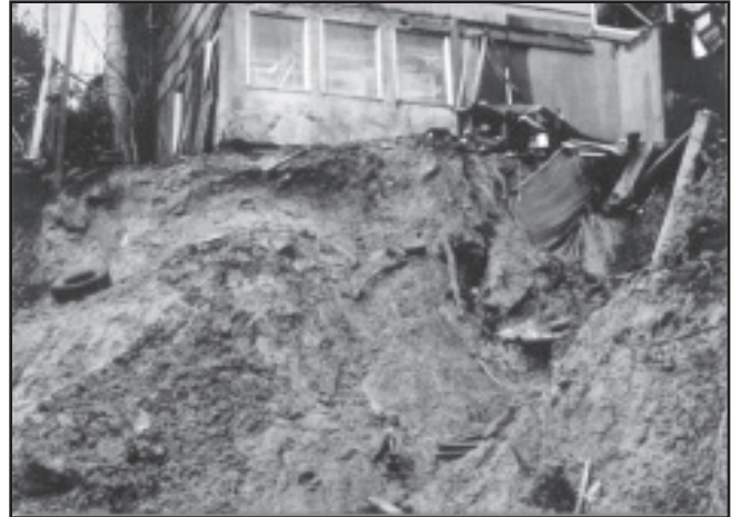
SDCI staff inspected nearly 400 private properties in Seattle for landslide damage after the 1997 New Year's Day storm.
