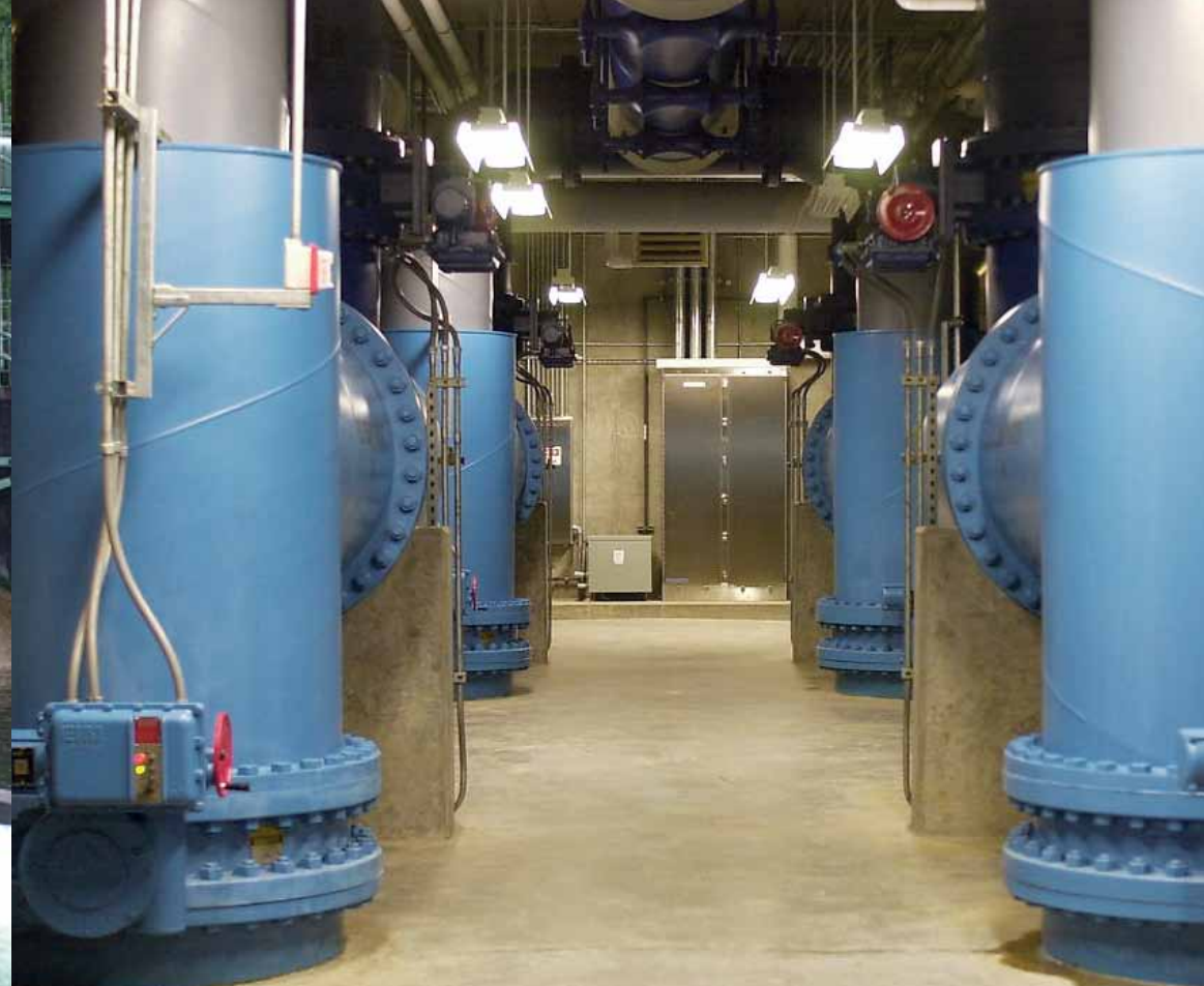
Tolt water treatment facility.
