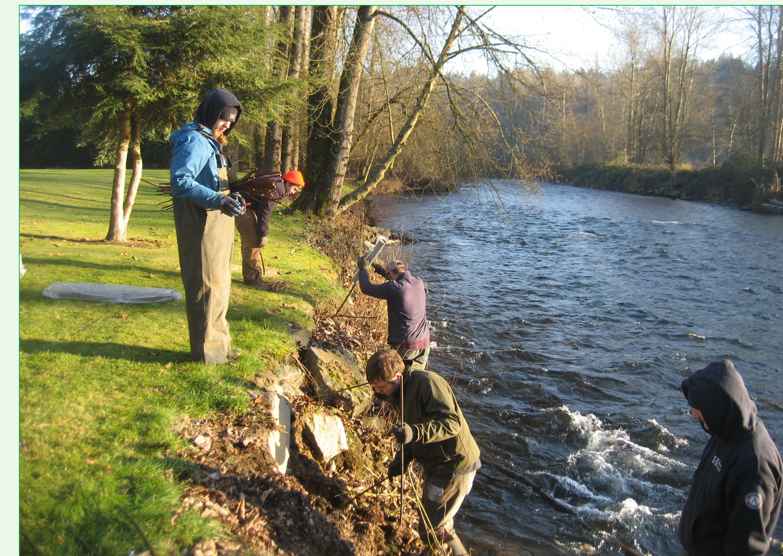
Crew installing plants at private site after treatment work has been conducted.
