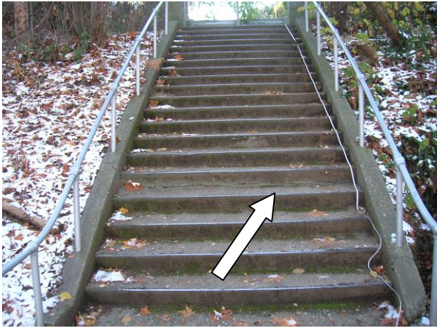
Figure 3. Cracking in the stairway
