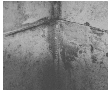
Figure 2. Mortar Patch for Spall Repair
