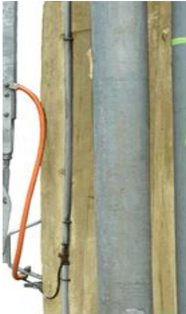
Figure 3.4 Switch Handle Grounding
