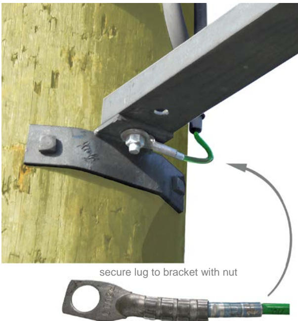
Figure 3.3c, Routing Ground Wire
