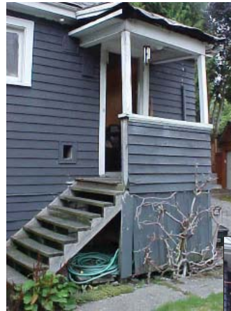
Before: rotting wood steps, no handrail for safety, unstable platform
