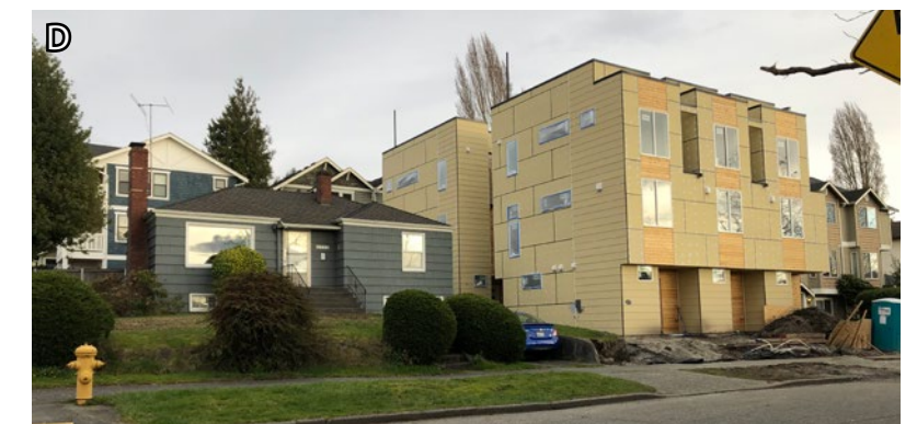
Townhomes New townhomes under construction with a modern aesthetic which speaks to the evolving character of the area.
