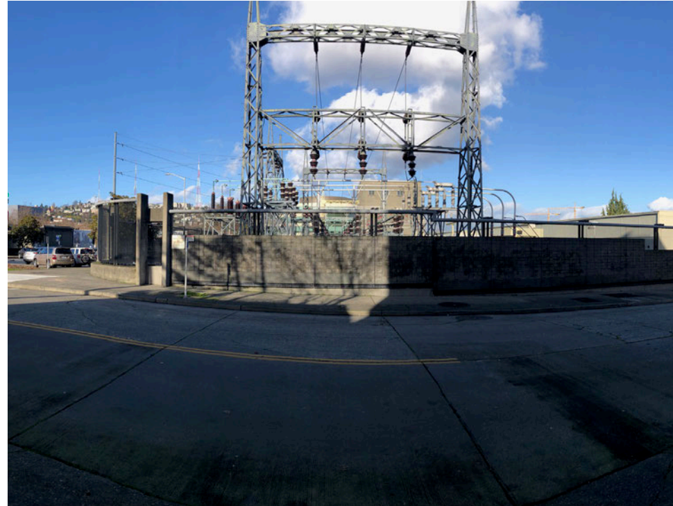
① SEATTLE CITY LIGHT BROAD STREET SUBSTATION 565 Harrison Street
