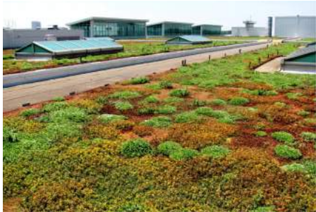
SEDUM BASED GREEN ROOF
