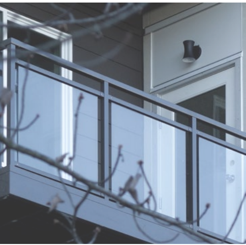
DC-4: Aluminum/glass guardrails
