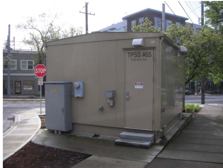
North side of street car electrical substation
