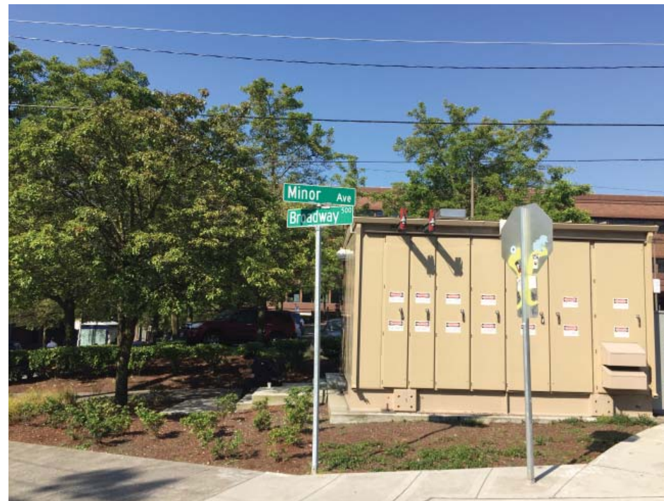
East side of streetcar electrical substation
