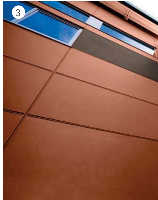
FIBER CEMENT PANEL COLOR: BM MAYFLOWER RED HC-49 ACCENT: BM BUREN BROWN HC-70
