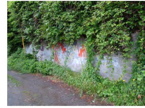
Existing block wall with grafiti on site
