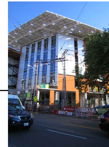
E MADISON LOOKING SW BULLIT CTR "LIVING BLDG" -OFFICE, ENTRY OFF MCGILVRA METAL SID'G
