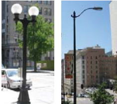
Existing standard street lighting poles
