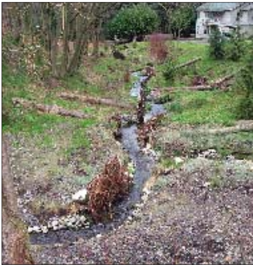
Restoration work along Willow Creek (south branch of Thornton Creek; photo courtesy Seattle Municipal Archives; photo by Toczek)
