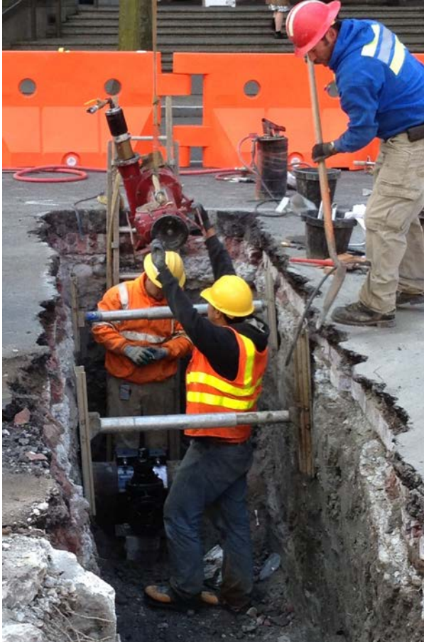
Water Taps or Service Installations
