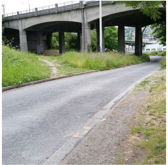
The 15th Ave W southbound onramp needs to be rebuilt
