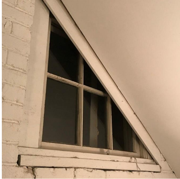
Figure 14) Photograph of extant window in the east façade at the second floor level of the subject building.
