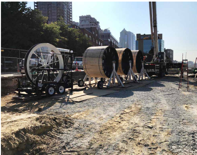
The spools of 115kV transmission line at the relocation site of Seattle's waterfront
