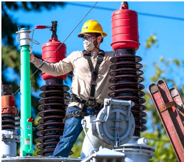
City Light's Max Romero atop a transformer. Photo credit: Hugo Ludeña. Artwork commissioned with Seattle City Light 1% for Art funds as part of the Essentially Seattle public art project.
