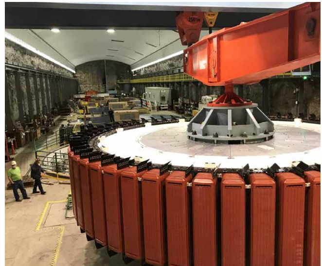
A new rotor at the Boundary Hydroelectric Project.
