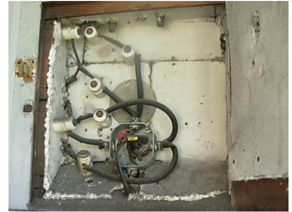
Code violation at Sisley property. Photo Credit: City of Seattle.
