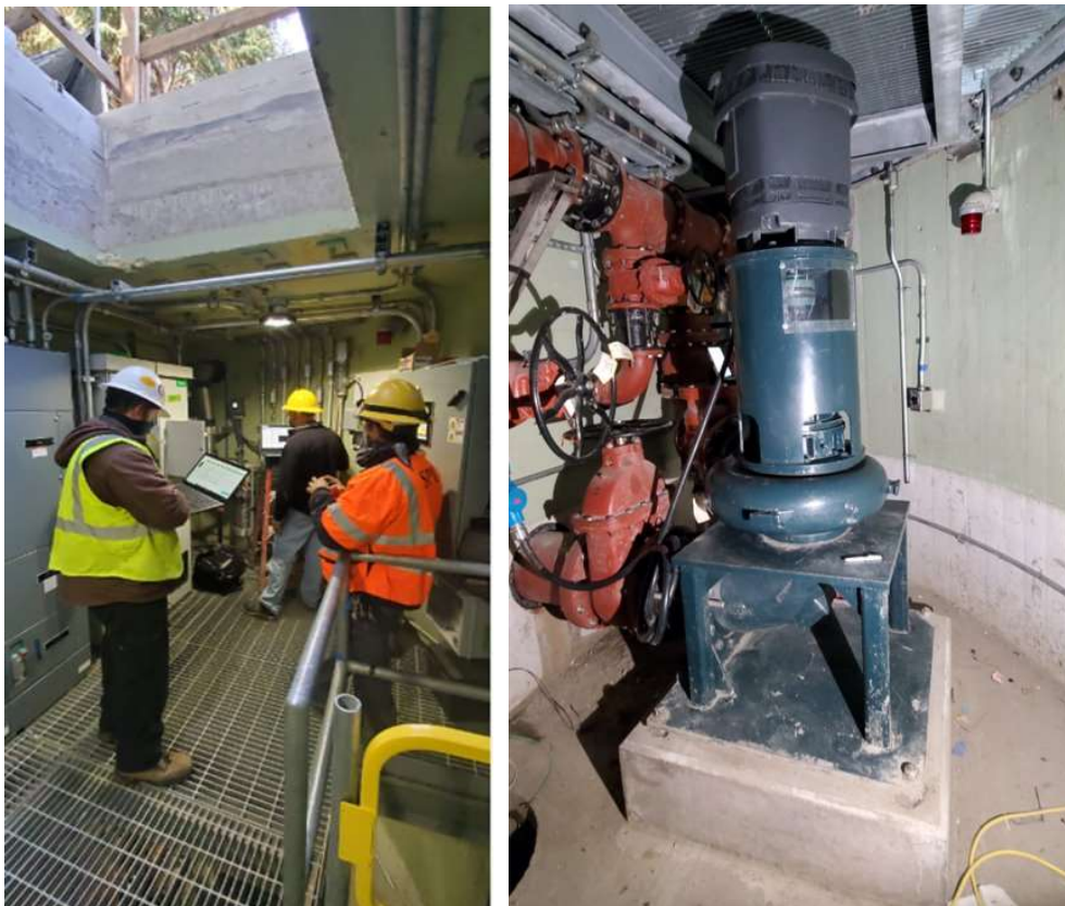
Figure 4-3. Operational Testing of Upgraded Pump Station 13 (left) and new pumps and valving (right)
