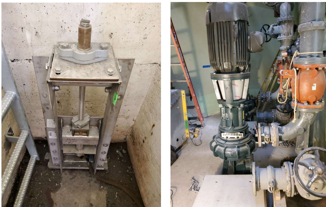
Figure 4-4. Installation of Basin 138 slide gate (left) and new higher capacity pumps (right)
