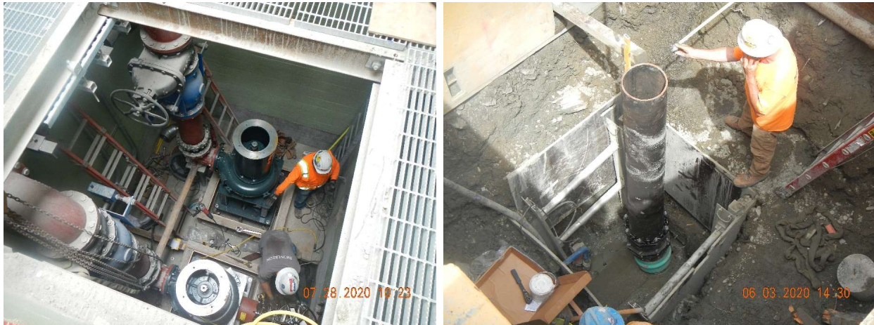
Figure 4-2. New Basin 60 pumps being installed (left) and New Basin 60 connection to King County trunk sewer (right)
