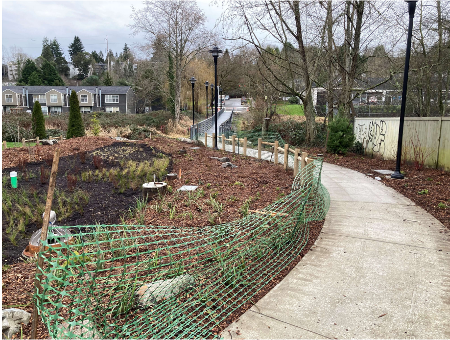
Figure 4-9. Looking east from 24 th Ave SW and SW Kenyon St – the new bioretention facility, walkway, and bridge
