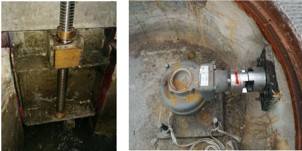
Figure 4-1. New Basin 99 Sluice Gate (left) and Actuator Motor (right)
