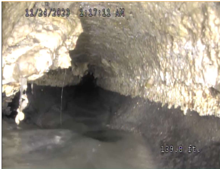
Figure 3-1. 2023 Mainline pipe demonstrating visible FOG accumulations
